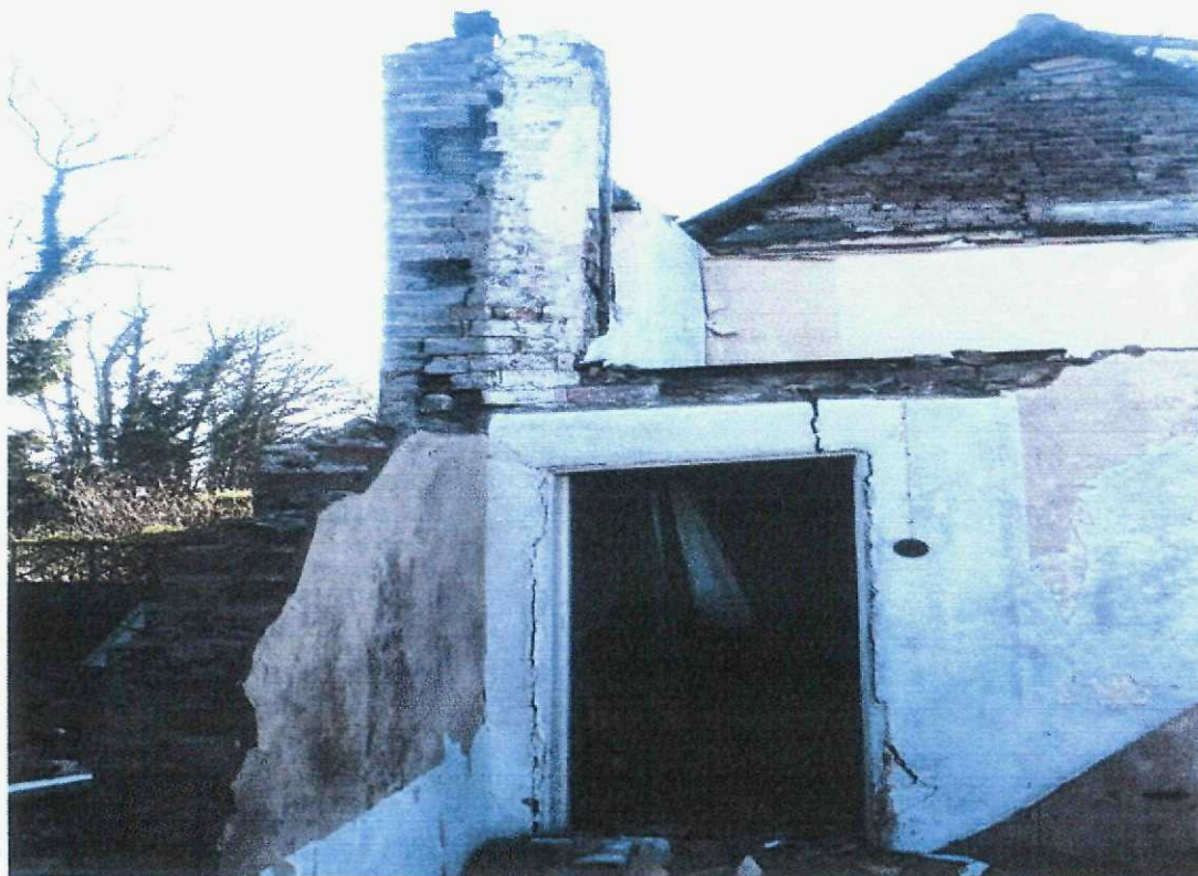
Plate 3 – View on end of wall showing vertical and lateral displacement
