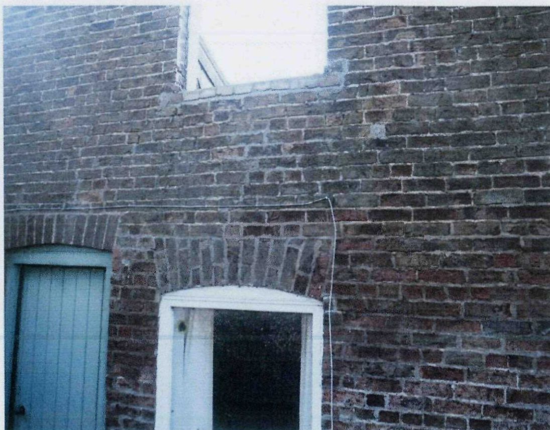
Plate 2 – Close up showing repointed cracking on front elevation
