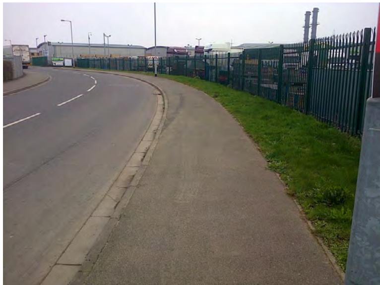
PHOTO 3: Tyre Marks on Footway on Southern Side of Bervor Close
