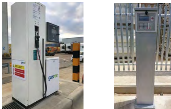
Figure 3.3 – Biomethane CNG Dispenser and Fuel Management Unit
