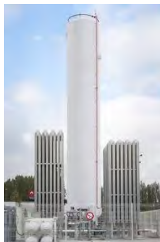
Figure 3.2 – Vertical LNG Storage Tank
