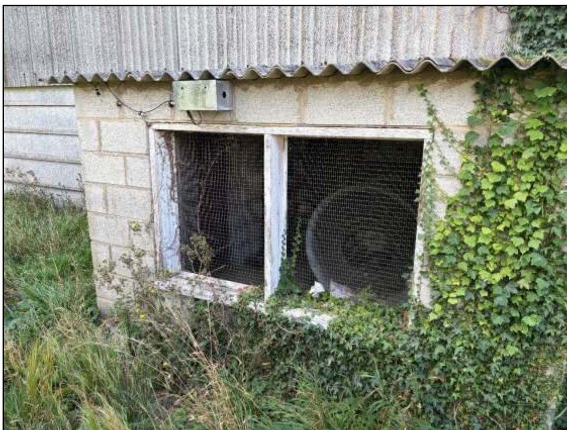
Fig 8 – housing for the electrical cooling fan
