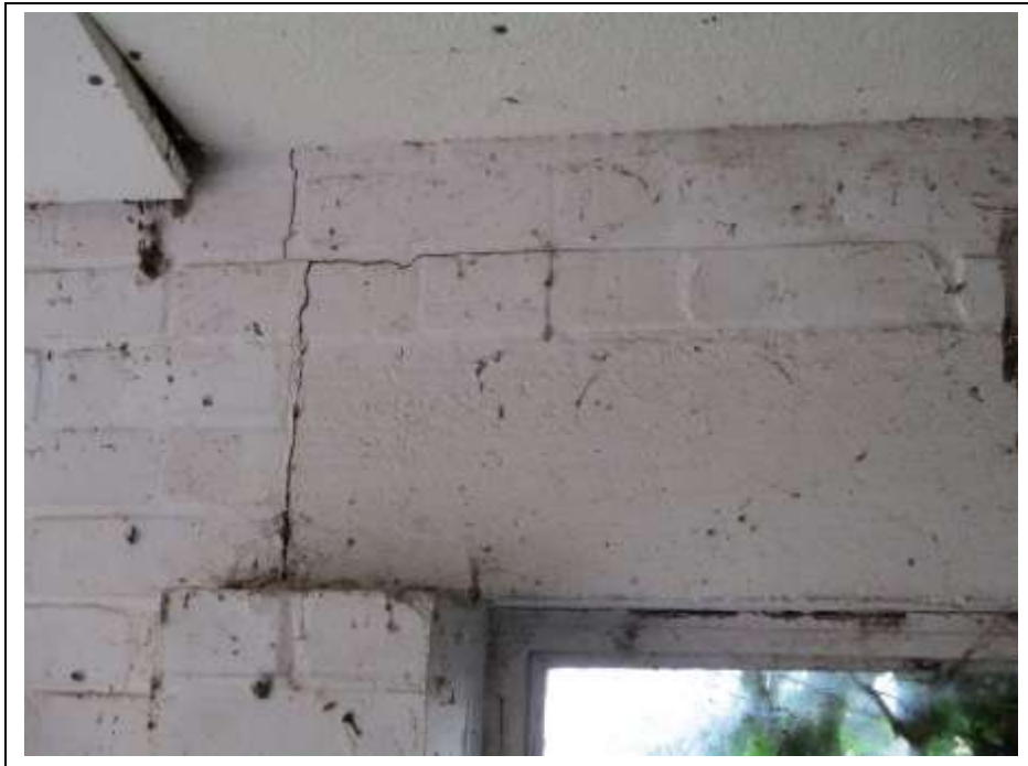
Plate 21. Minor cracking in entrance.
