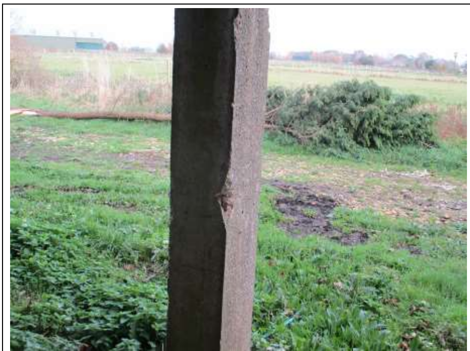
Plate 12. Minor spalling to concrete.
