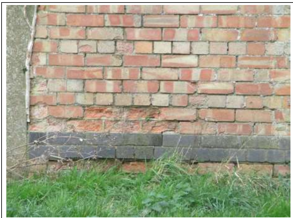
Plate 14. Localised wear and tear.
