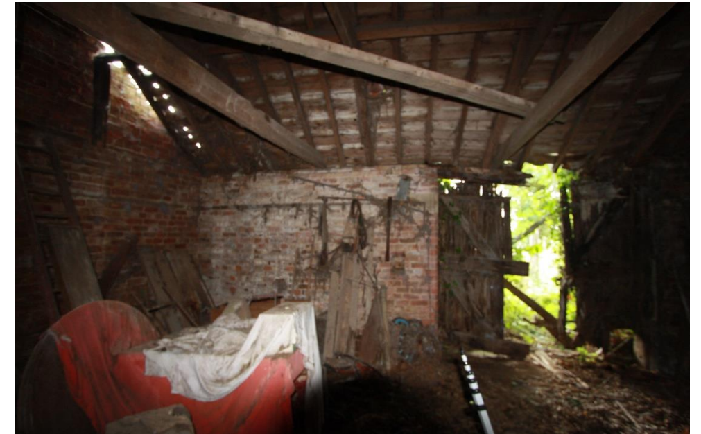
Image illustrating the damage to the roof structure above the double doors at the gable verge due to the failure of rainwater goods
