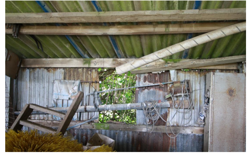
Image illustrating damage to metal corrugated sheeting
