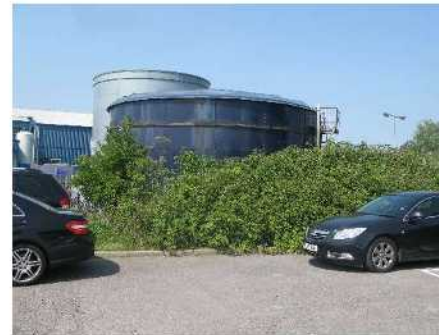
Effluent tanks seen from staff car park
