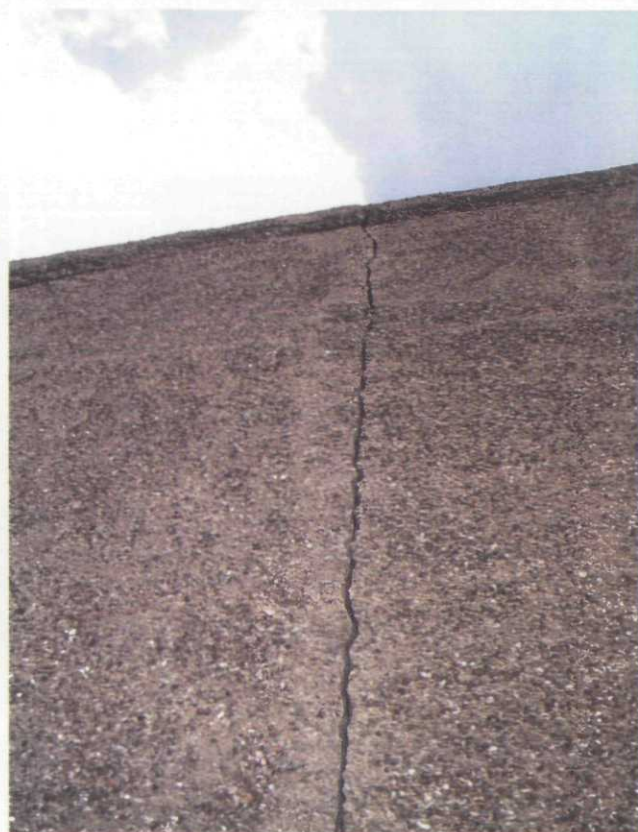
Name: IMGP1733 Date: 20/05/2004 16:43:30 Description: Left hand elevation, vertical cracking/differential settlement
