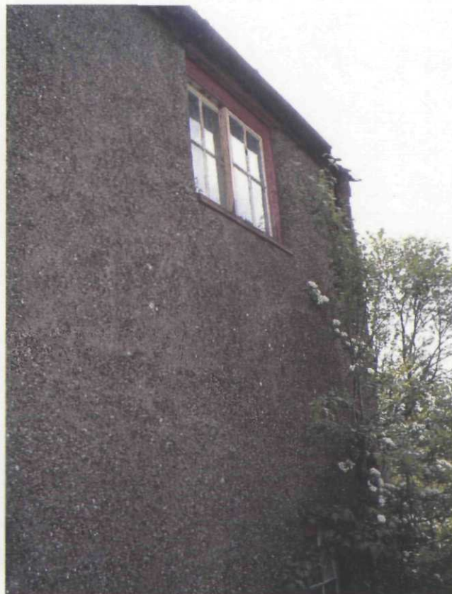
Name: IMGP1731 Date: 20/05/2004 16:43:09 Description: Cracking at rear left hand corner
