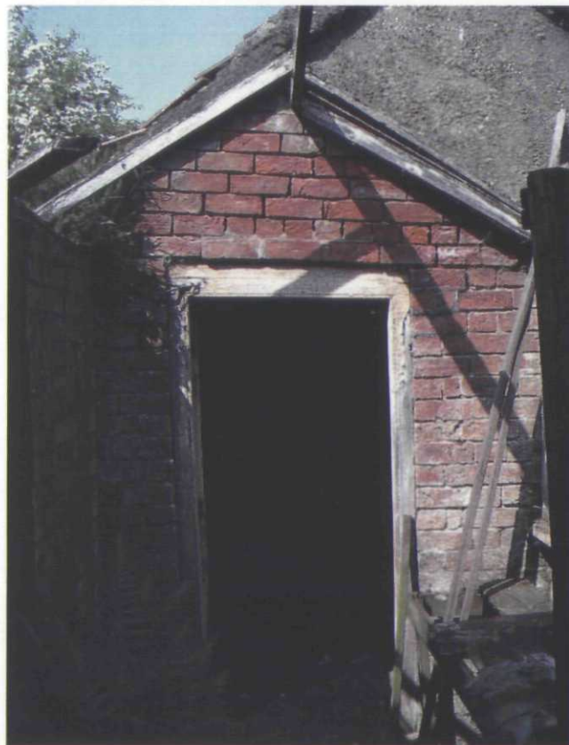
Name: IMGP1730 Date: 20/05/2004 16:43:02 Description: Rear elevation, distortion to kitchen/outhouse
