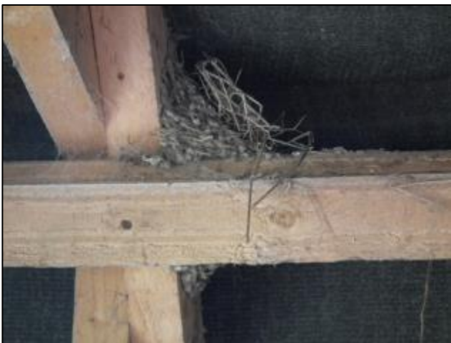
Fig 22: Evidence that the buildings are used by birds for nesting
