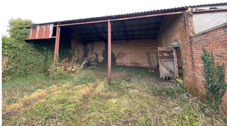
The open section will require a new floor
