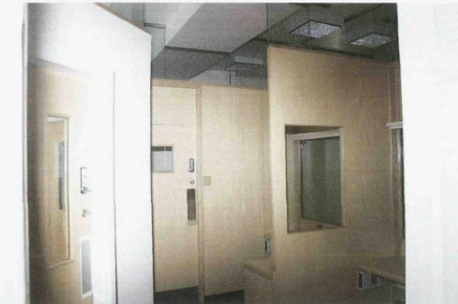
Plate 17: Modern partitions cluttering the front north-east ground-floor room
