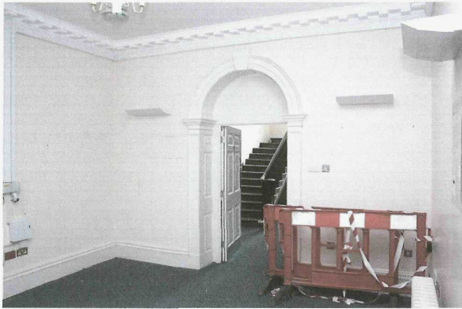
Plate 14: The entrance hall and arched opening with inappropriate infill
