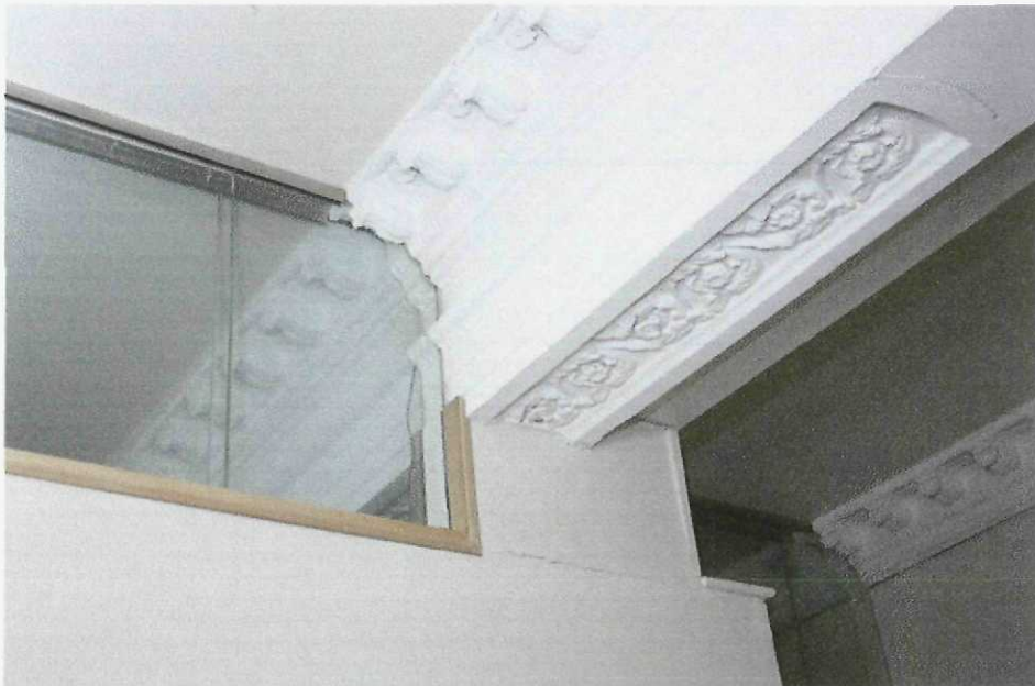
Plate 21: Front south-west room: modern partition needlessly cut into the cornice.
