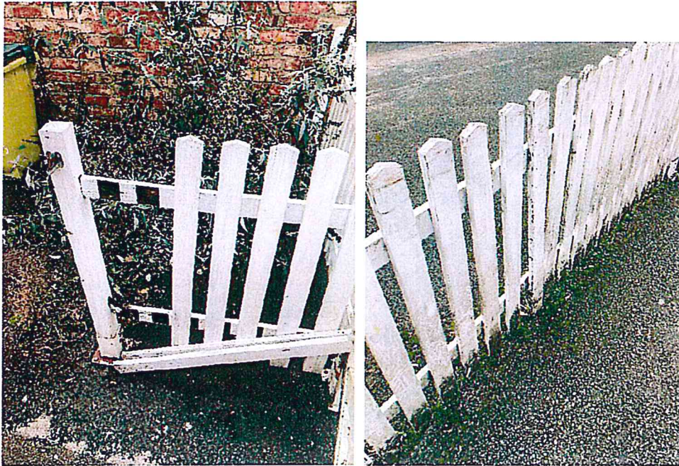
Gates and picket fencing flimsy and posts rotten at the base
