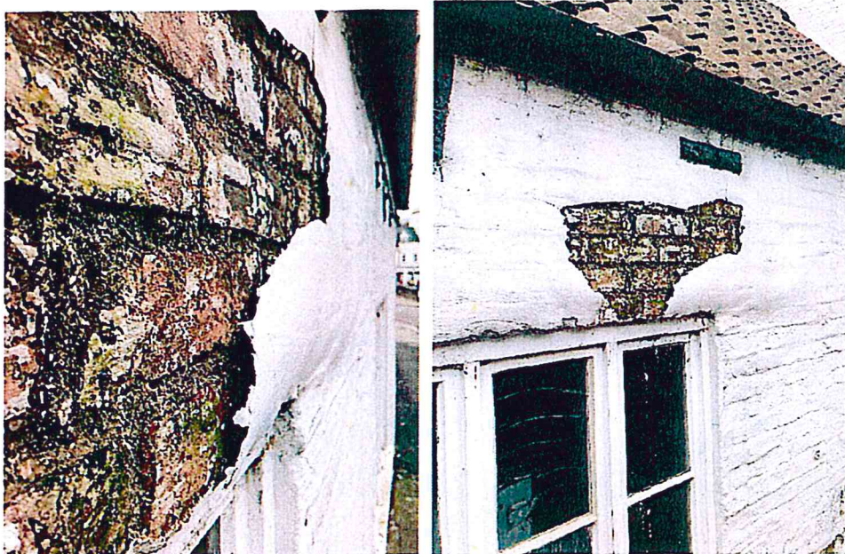
Paint blown from bricks
