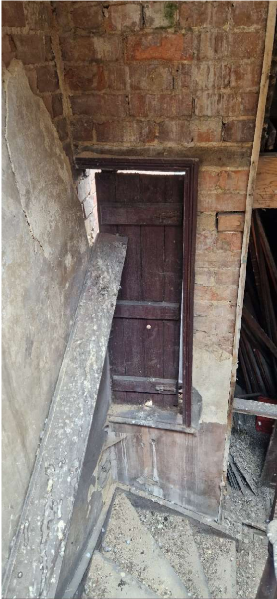
Hatch at first floor level with gaps between panel and frame
