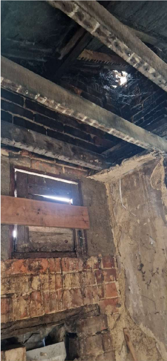
Hole at high level in roof and hatch below with gaps between panel and frame
