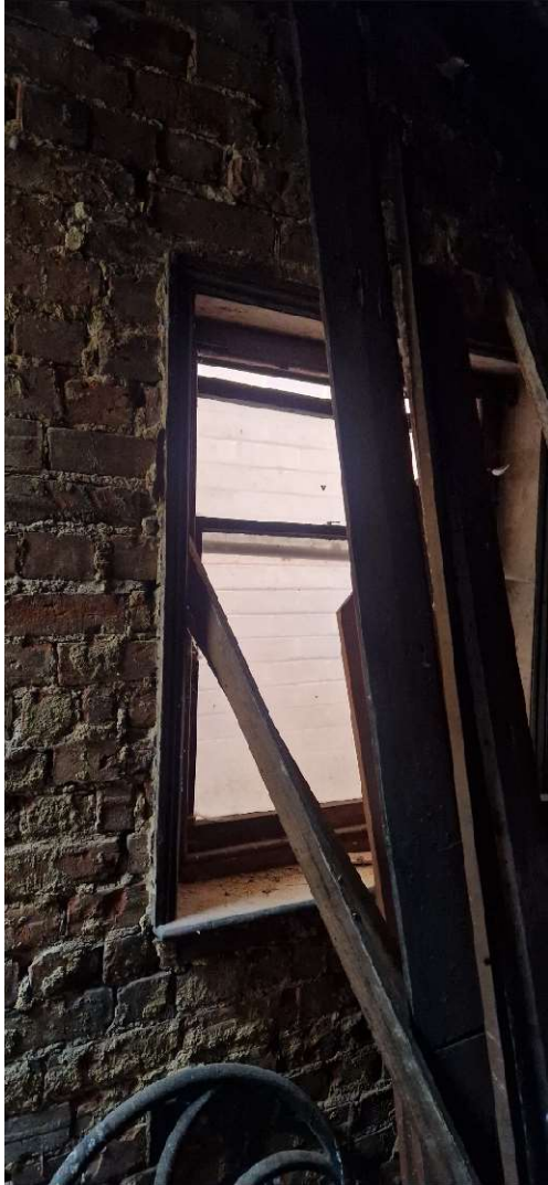
Slightly open window at first floor level
