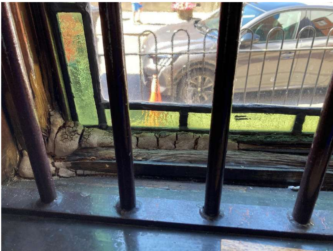
Detail of rotten window frame on right-hand side of entrance
