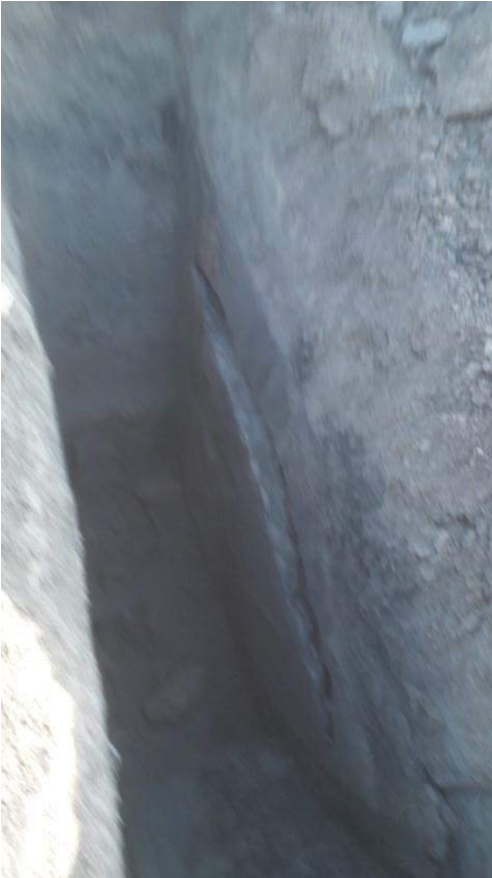
TP103, just prior to collapse of side.
