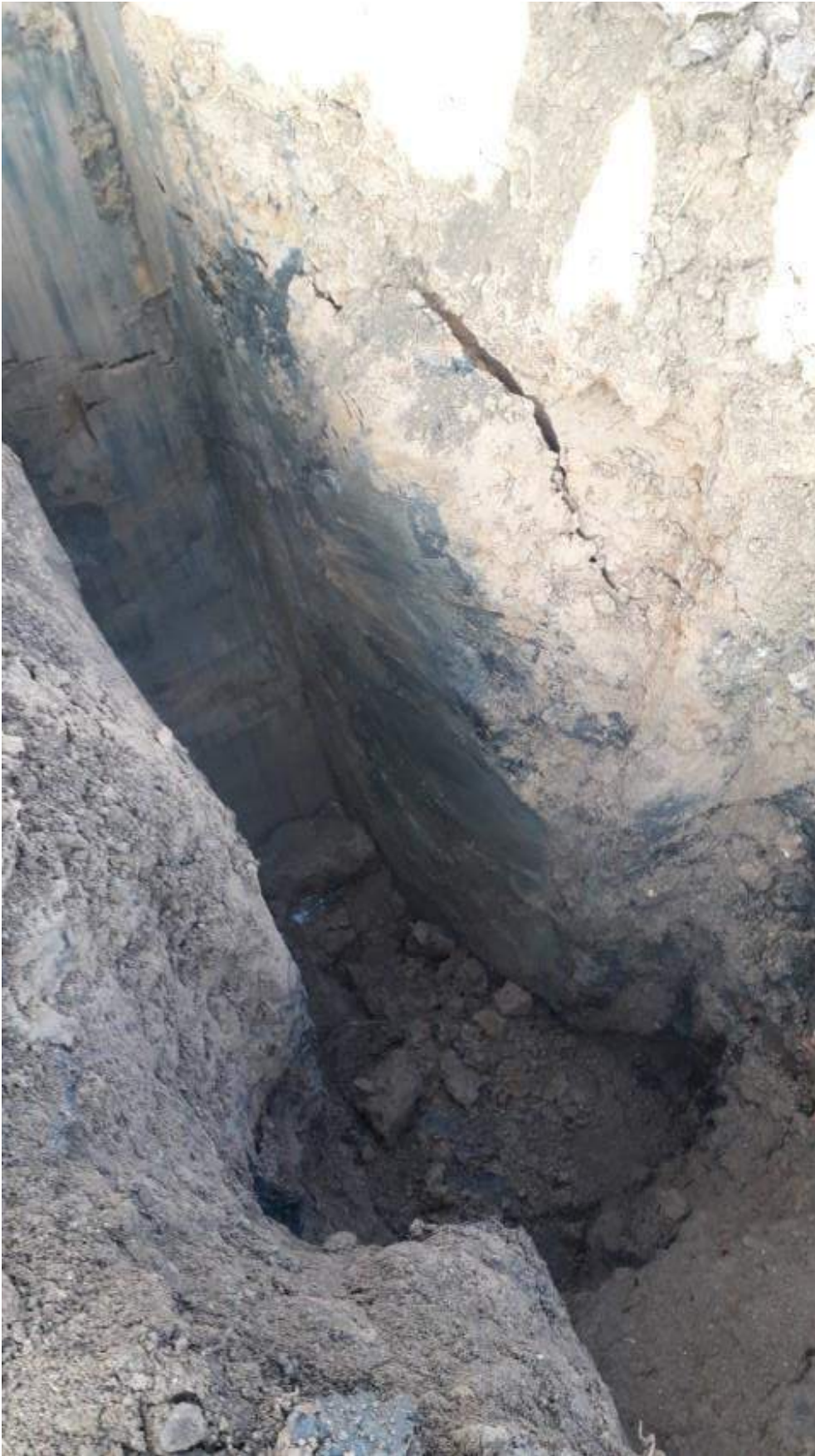
TP100. Prior to complete collapse.
