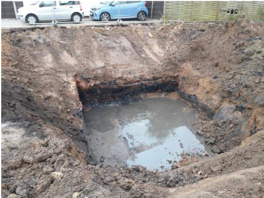
View looking west across exposed cradle. The cradle brick walls are visible at the rear and along the sides. The walls are in poor condition, with collapse noted locally.
