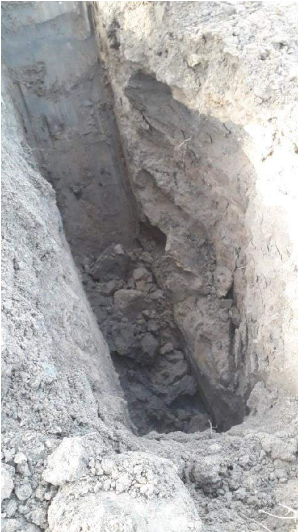
TP107 on completion. Some side instability evident.
