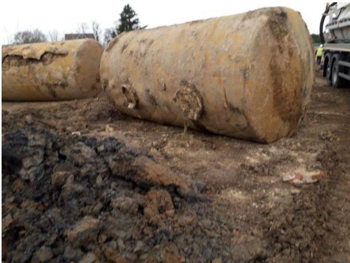
Close up of the tanks. Each has two access points (one for each compartment).
