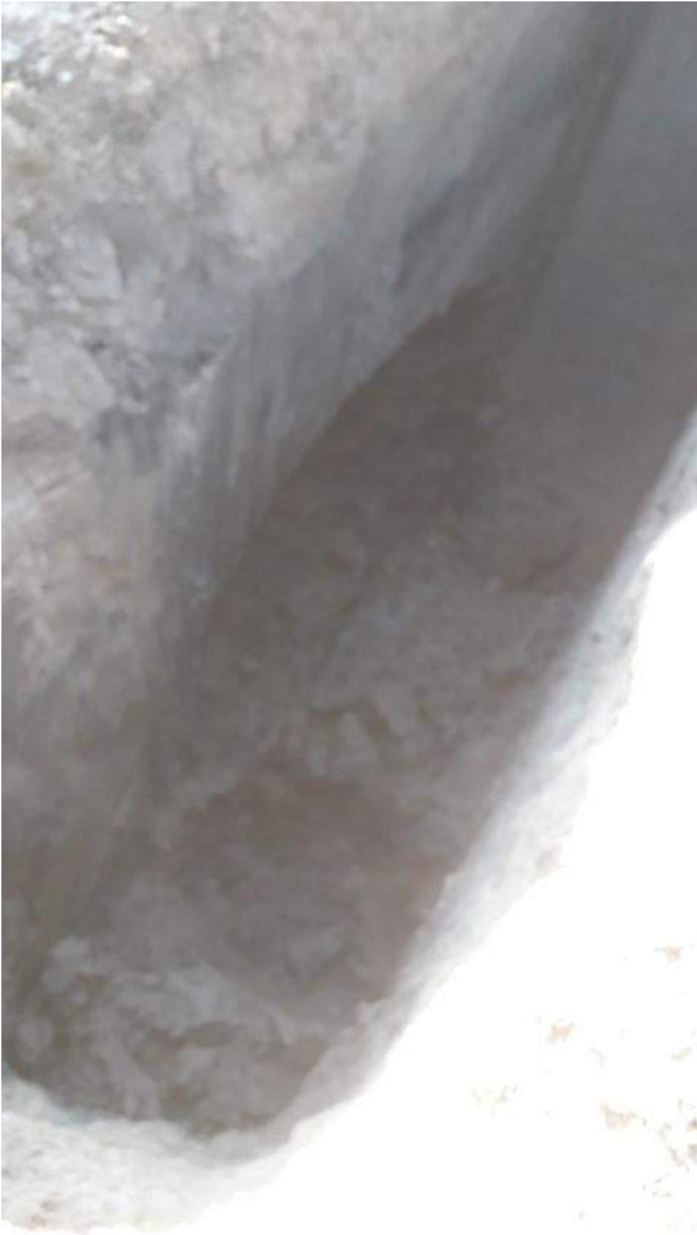
TP102, showing collapse at around the water table/seepages.
