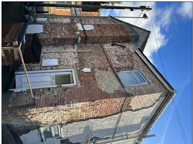
Area to be demolished due to movement & cracking
