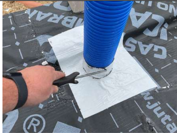
Plot 1. Pick & probe test to sealed pipe penetration's.
