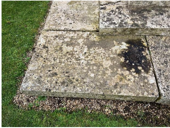
Fig 14 Damage and erosion to step surface.
