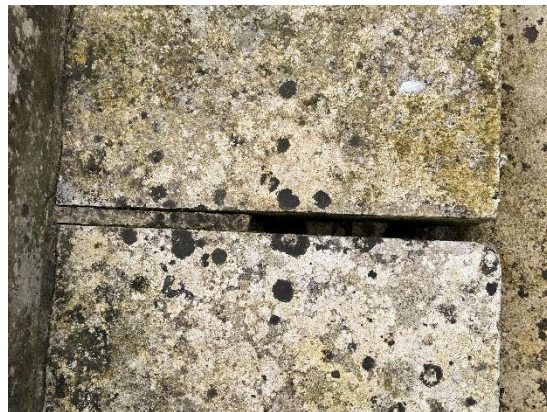
Fig 11 Mortar erosion in joint between slabs.
