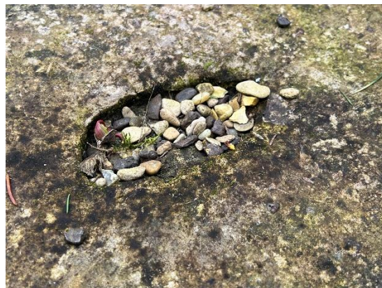
Fig 13 Damage and erosion to step surface.
