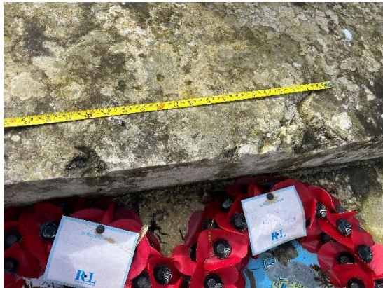
Fig 16 Damage to aris of step.
