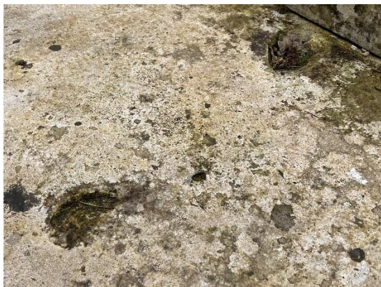
Fig 12 Damage and erosion to step surface.
