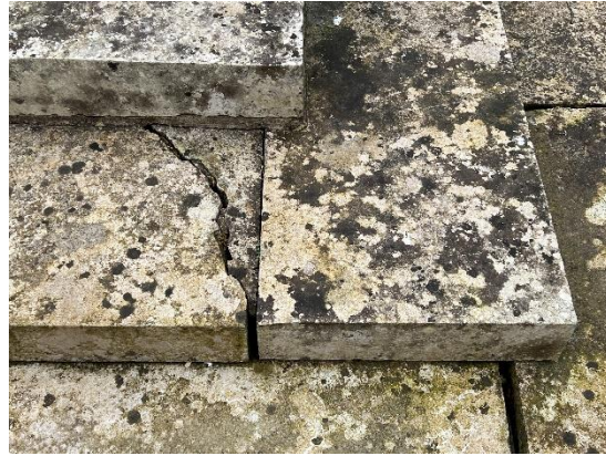
Fig 9 Crack through stone slab of step.
