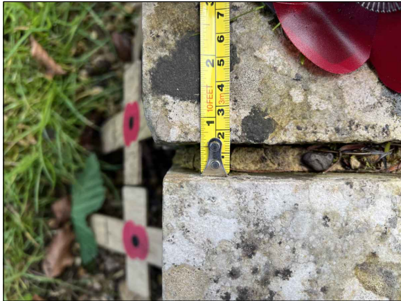
Photo 10 - Joint with pointing missing / eroded
