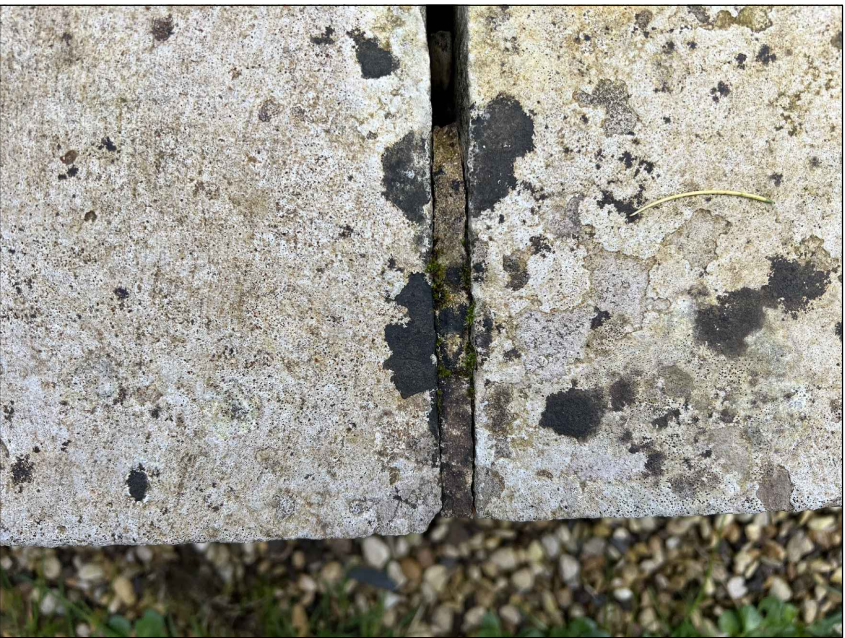
Photo 1 - Joint with pointing missing and vegetation
