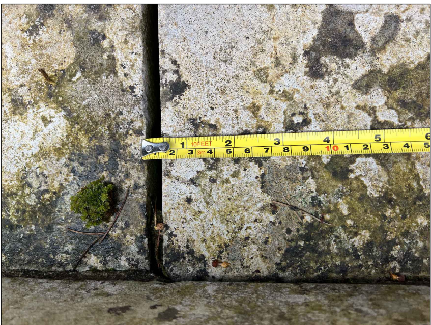
Photo 11 - Algae growth on stone surfaces, pointing missing.
