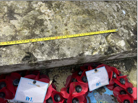
Photo 8 - Depressions and damaged arris to stone
