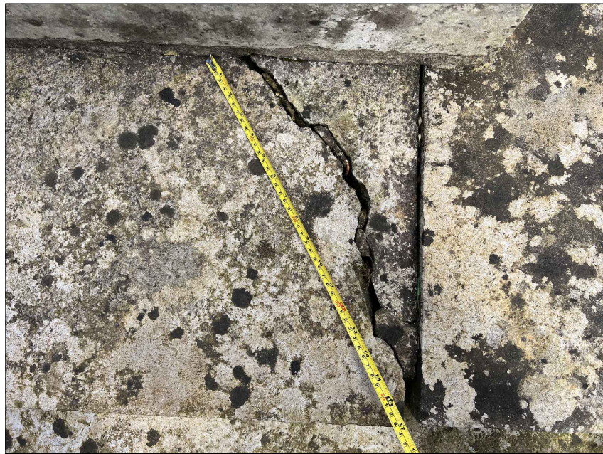
Photo 5 - Nominal 400mm crack through stone
