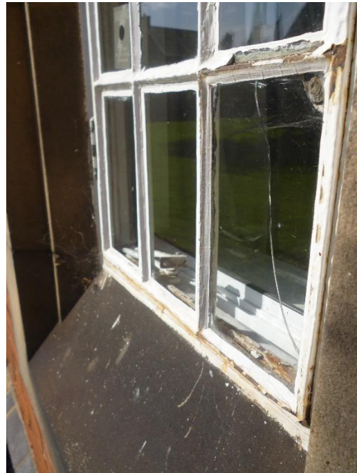
Debonding putty, cracked glazing and corroding frame.
