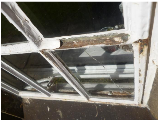
Debonding putty, cracked glazing and corroding frame.
