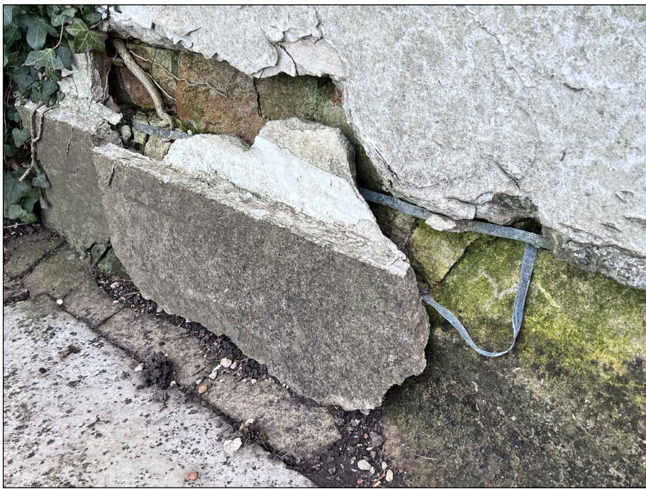
Image of eroded skirting detail
