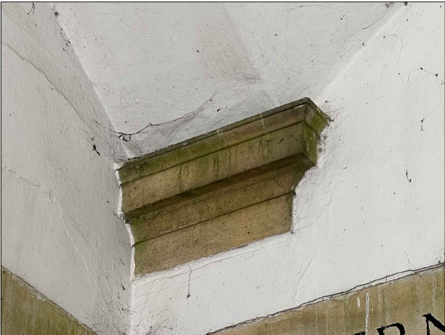
Heavily discoloured Corbel stone
