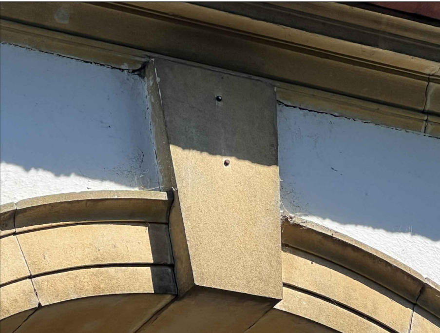
Removed fixing marks on keystones (typical)
