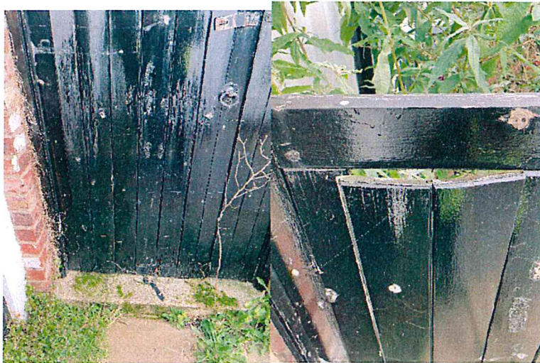
Replacement rear gate required, rotten at the bottom
