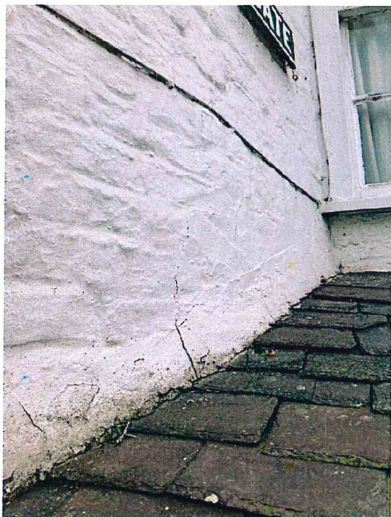
Cracking above collision point
