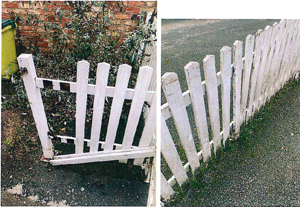
Gates and picket fencing flimsy and posts rotten at the base
