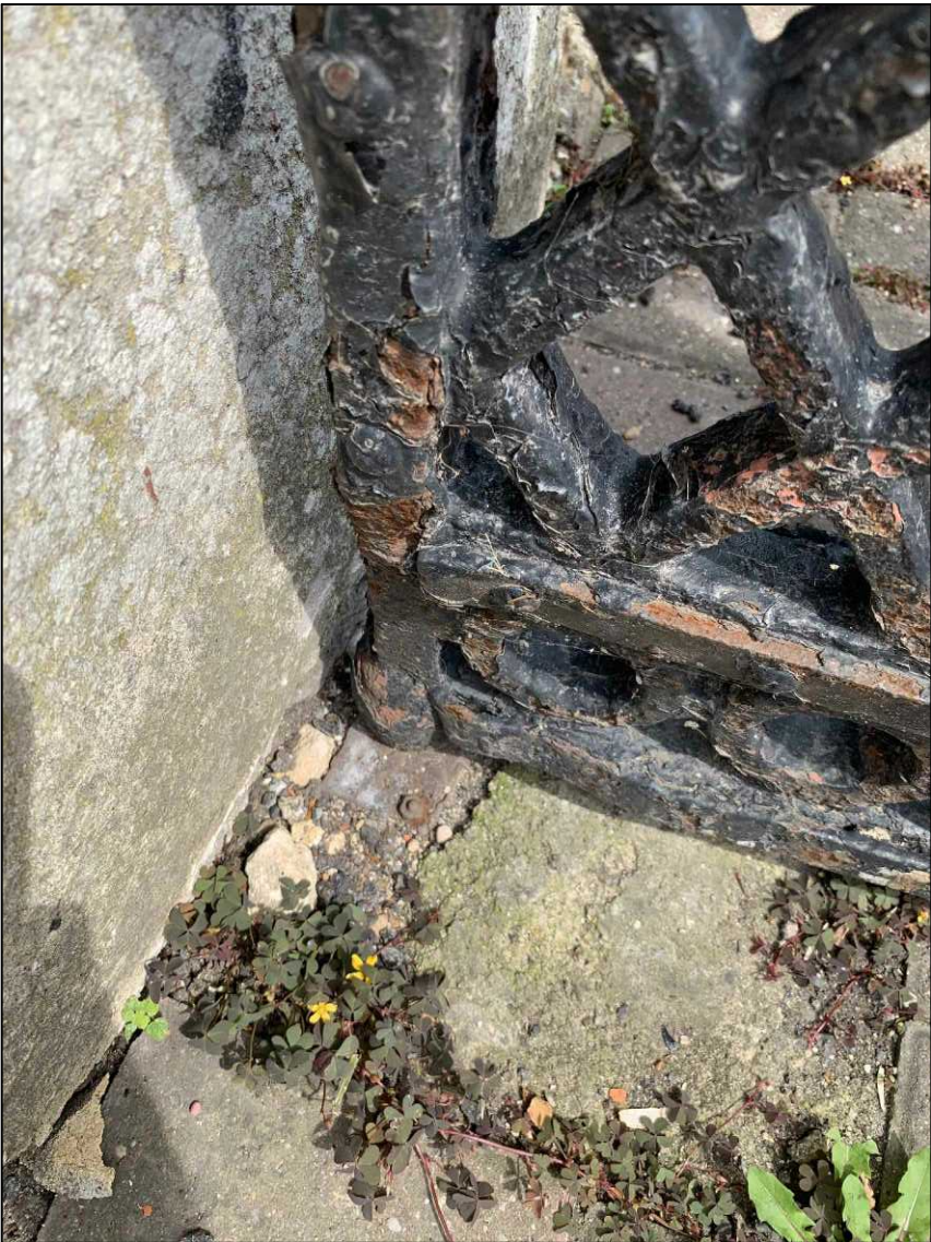
Ground-mount pivot point at north pillar
