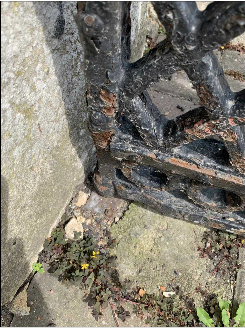
Ground-mount pivot point at north pillar
