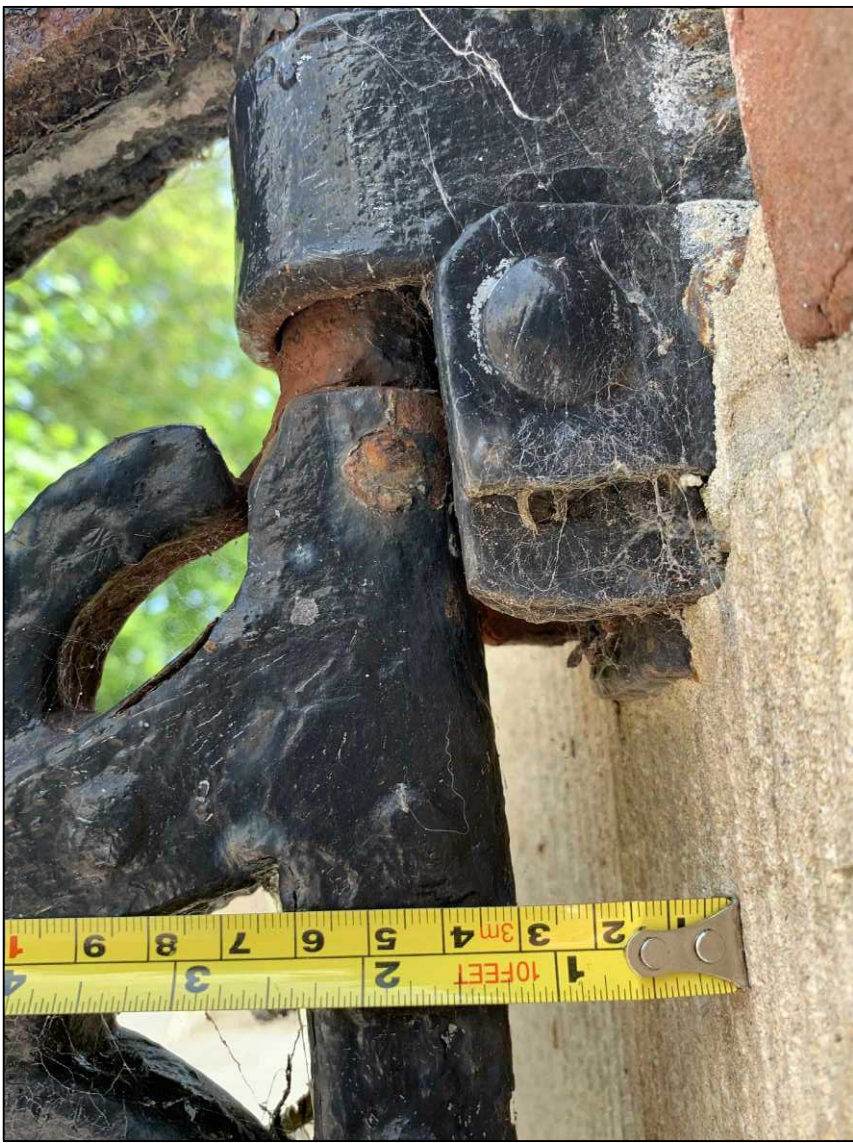
Fixed hinge point on south pillar
