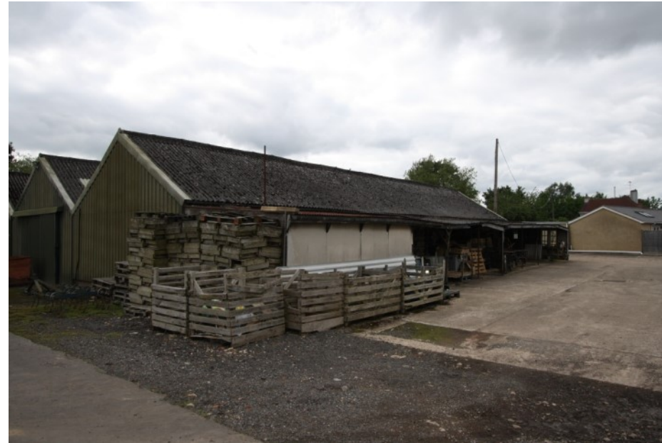
Dilapidated Lean-To to Existing Barn
