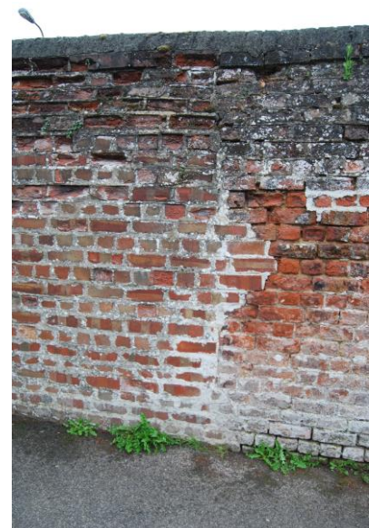
Fig 7. General Photograph showing the condition of the internal face of the boundary wall to the left of the gates where the battered face changes from four to five courses
