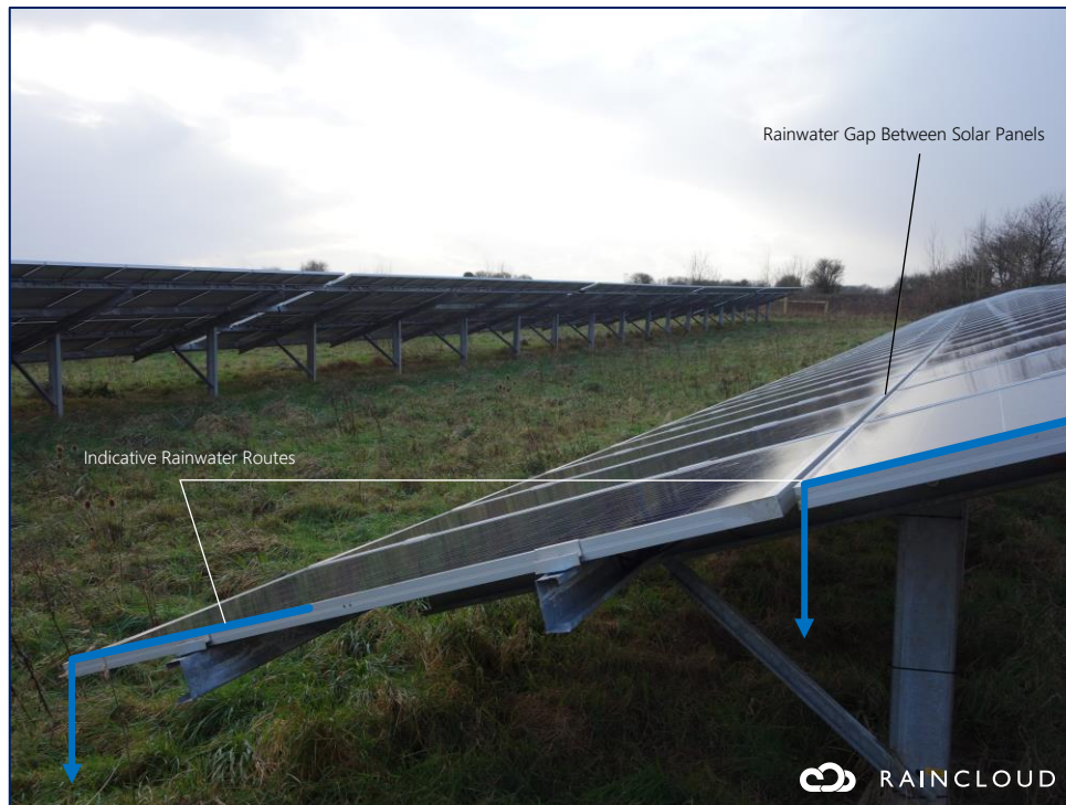
Plate 12: Rainwater gaps on PV array table
