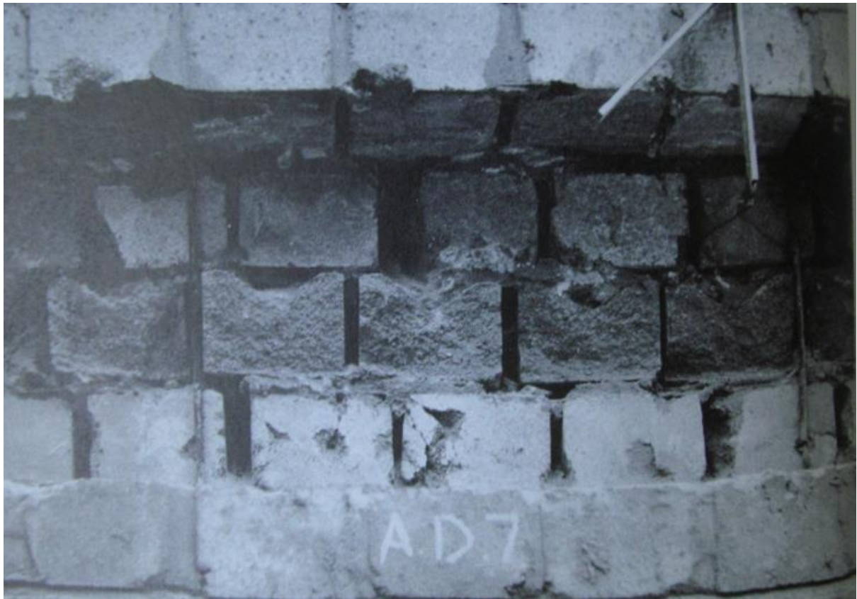
Historical Plate 19: Poor workmanship in brickwork on a surface air raid shelter, showing reinforcing bars (Source: Wade 2011: 40)
