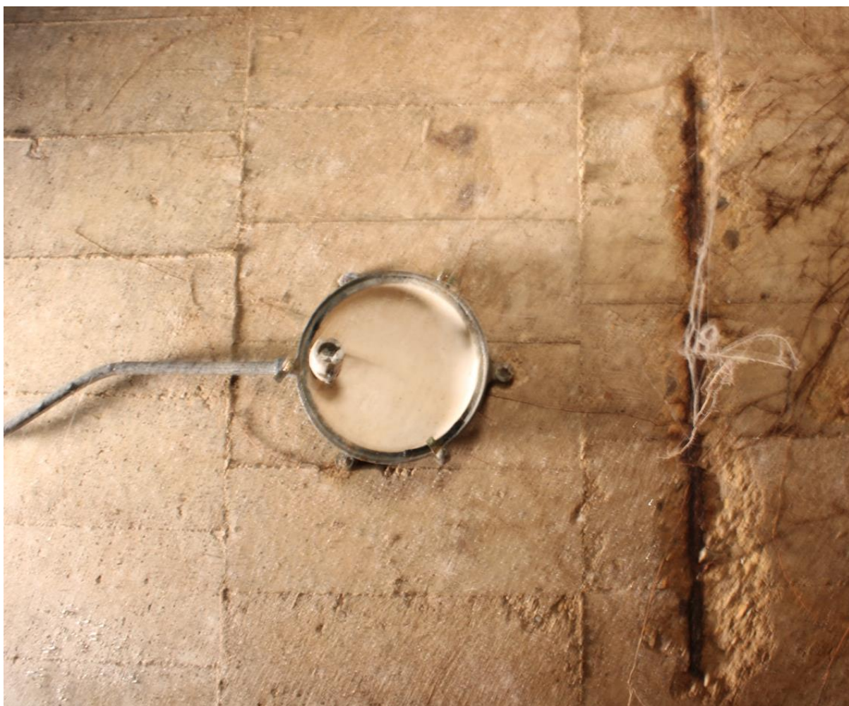
Plate 69: Ceiling light fitting at the south end of the shelter. This would have illuminated the area inside the south entrance to the building IMG_1585
