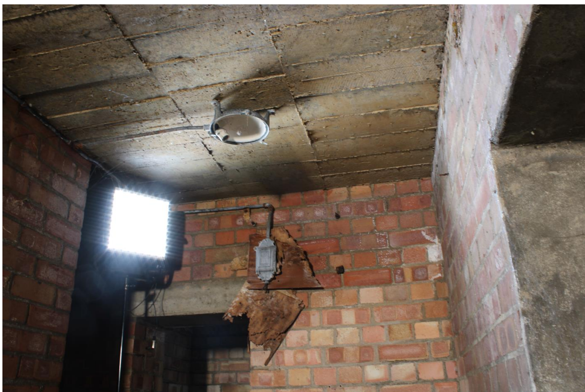
Plate 65: Junction box and board at northern end of east compartment, showing in-situ ceiling light fitting IMG_1562
