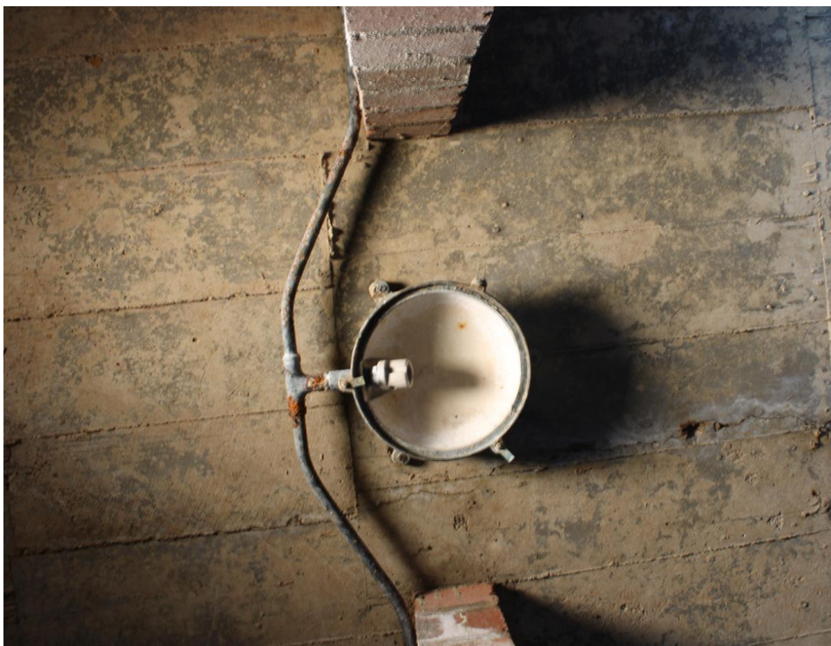
Plate 68: Detail view of central light fitting, showing method of attachment for bulb IMG_1576
