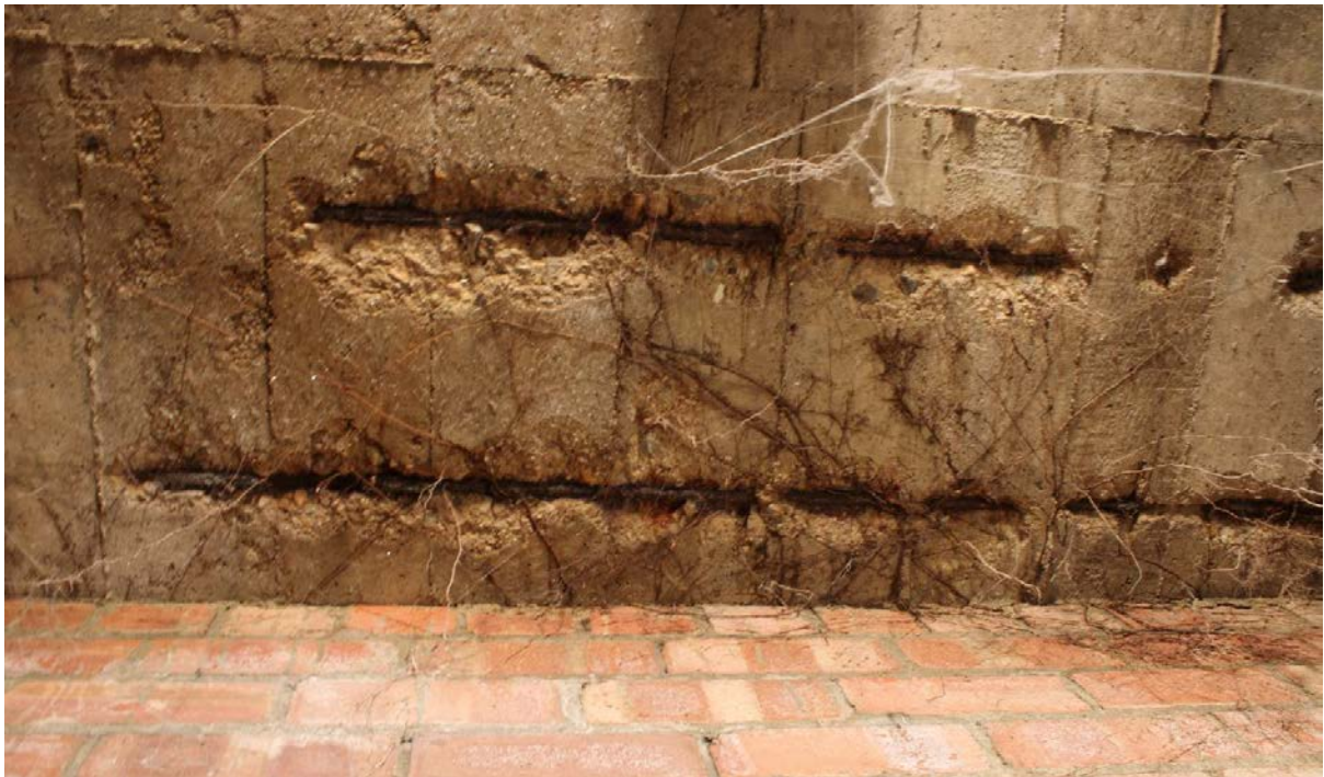
Plate 63: Exposed longitudinal metal reinforcing bars in the concrete roof slab IMG_1586
