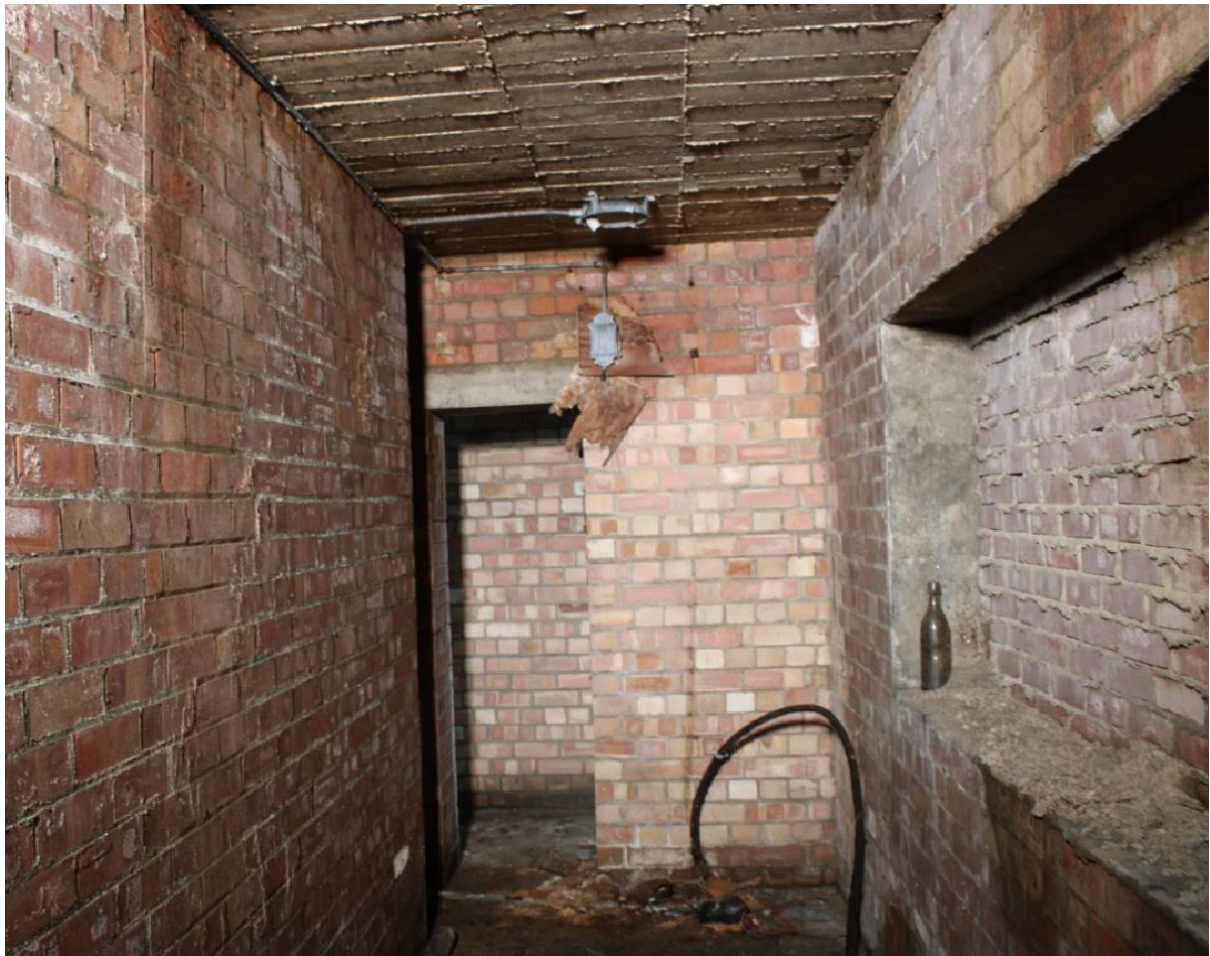
Plate 64: North end of the eastern compartment of the shelter, showing the mains electricity cable (bottom right). The high-level fuse board and a junction box can be seen above the lintel of the inner (north) entrance IMG_1548
