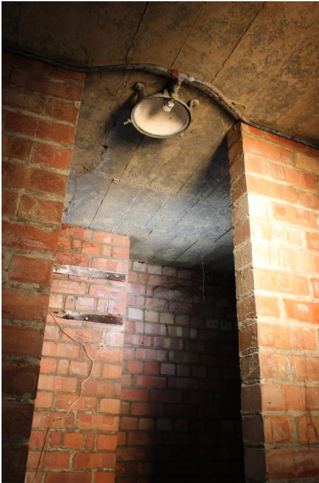
Plate 66: Ceiling light fitting in the centre of the shelter, illuminating both east and west shelter compartments IMG_1570
