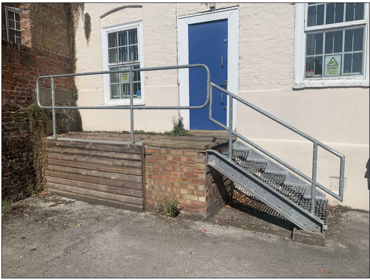
Rear landing, stairs and guarding to be repaired.
