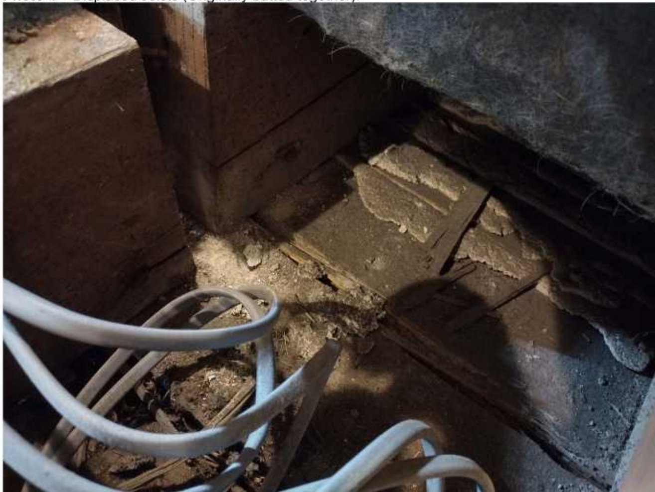
Photo 4 – Displaced Joists (Originally butted together):
