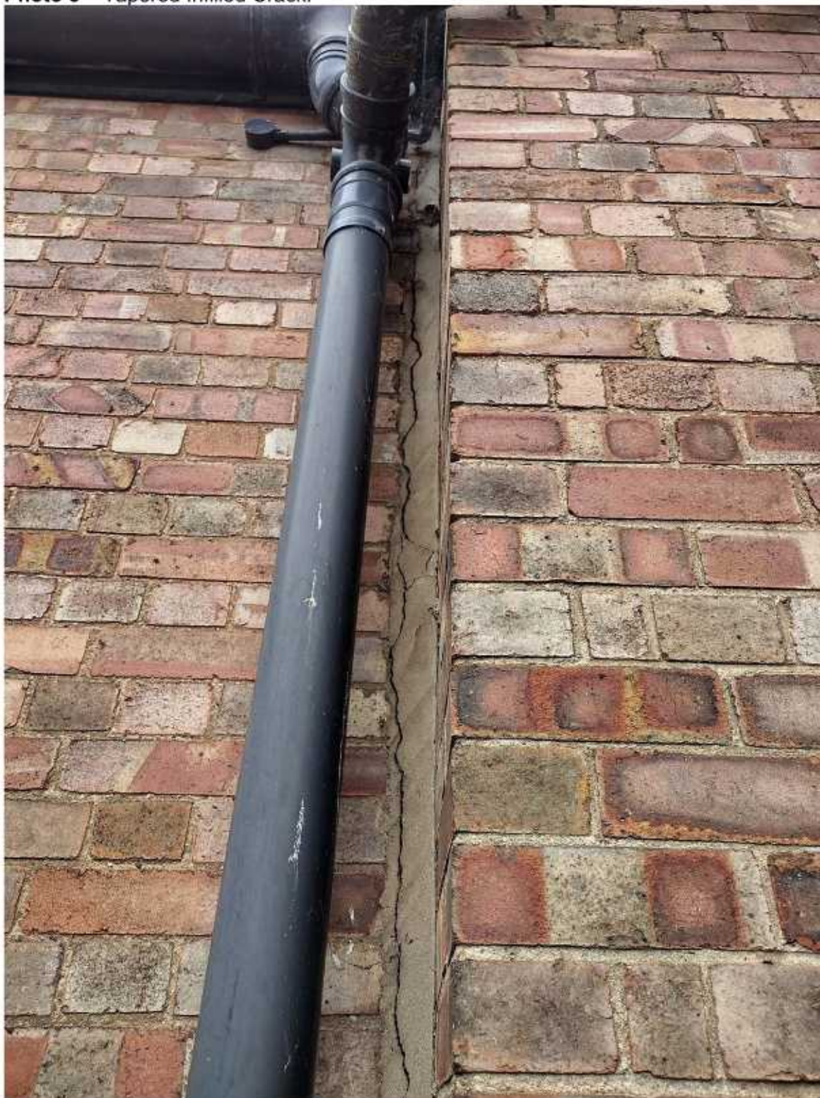
Photo 5 – Tapered Infilled Crack:
