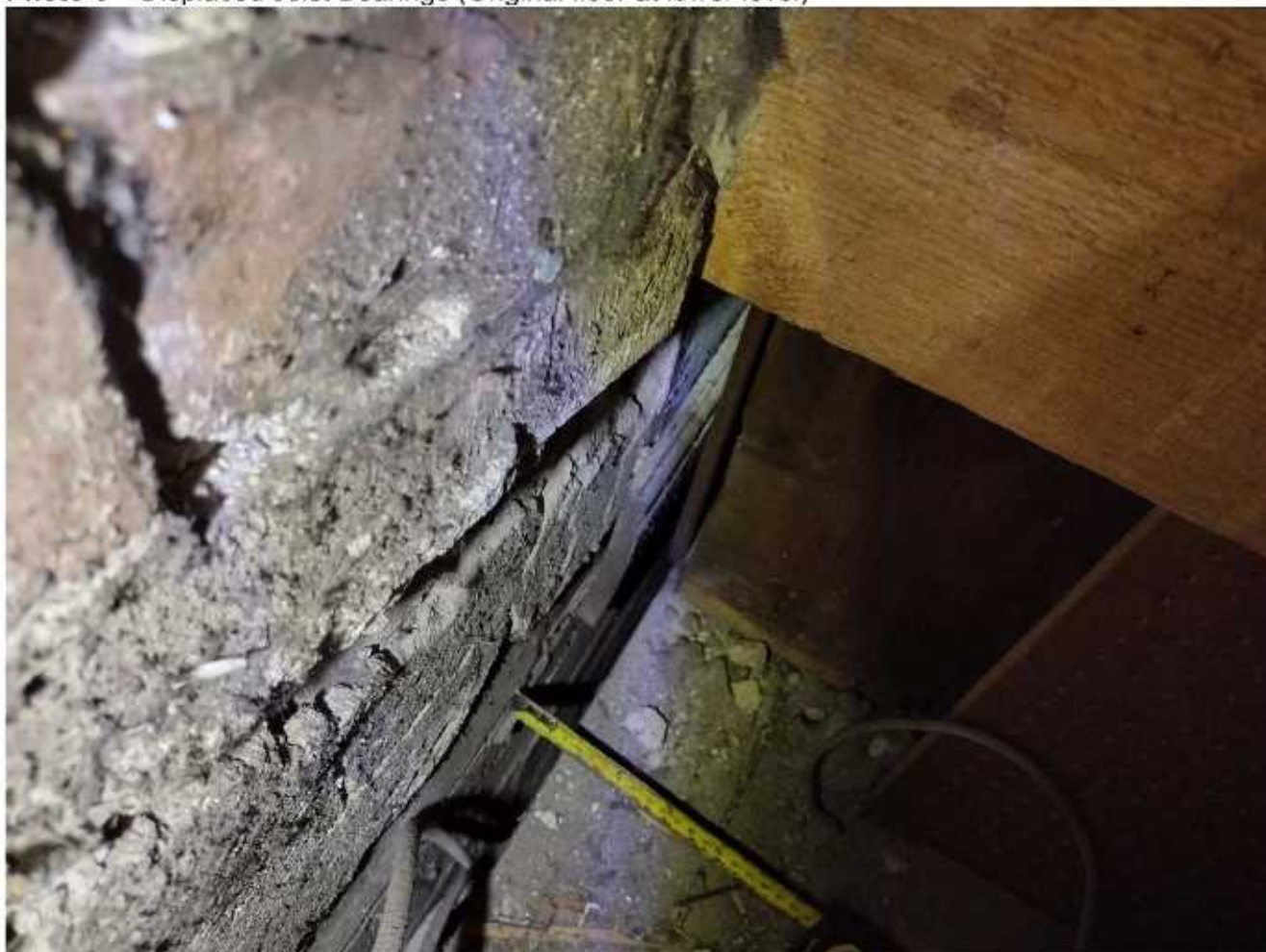
Photo 6 – Displaced Joist Bearings (Original floor at lower level)
