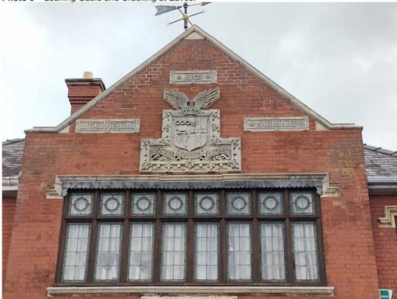
Photo 3 – Leaning Gable and Cracking at Eaves:
