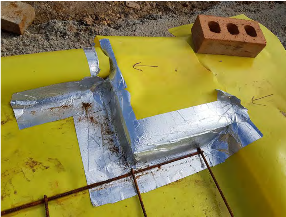
Photo 8 – Detail of defects identified in seal for Plot 926.
