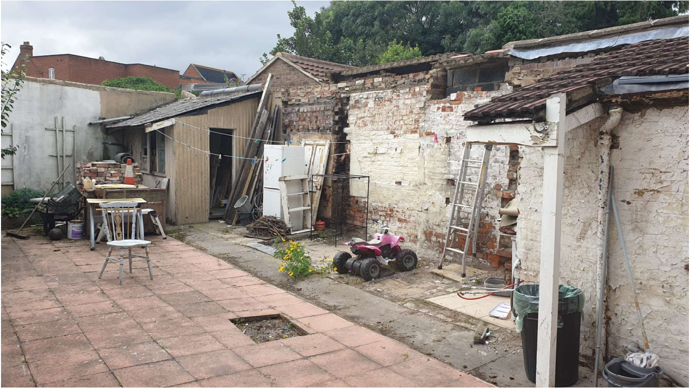
Images 2b. The existing rear of the property showing the current state of dilapidation.
