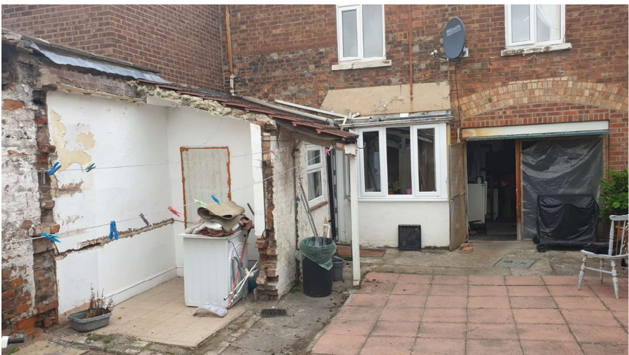
Images 2a. The existing rear of the property showing the current state of dilapidation.
