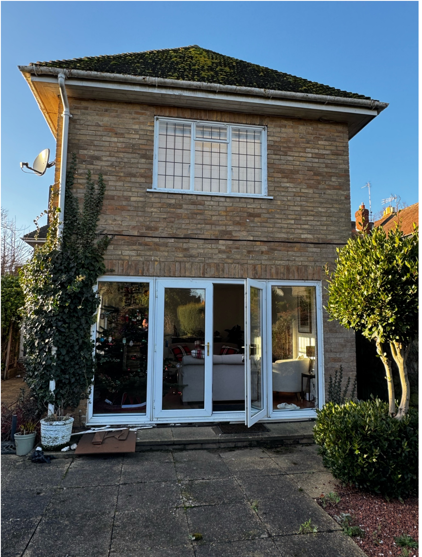
Rear side elevation. All eight windows to be replaced and French door.
