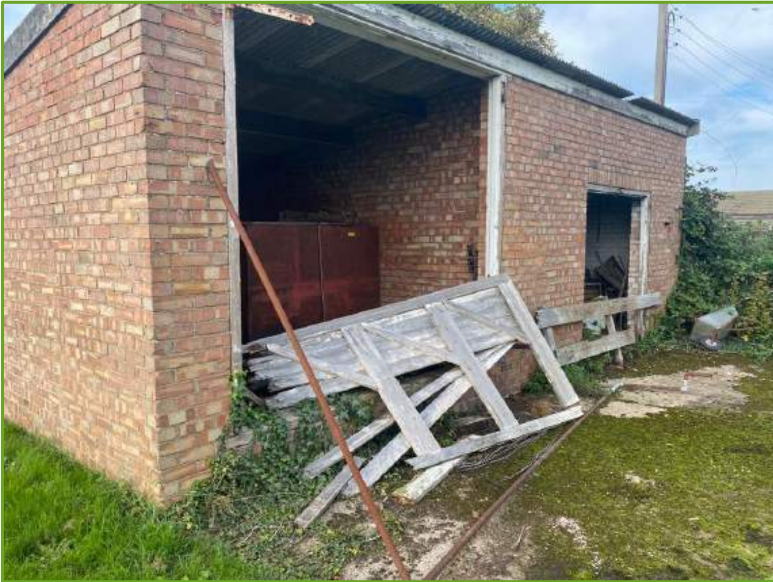
Photograph 5: Northern outbuilding - derelict.
