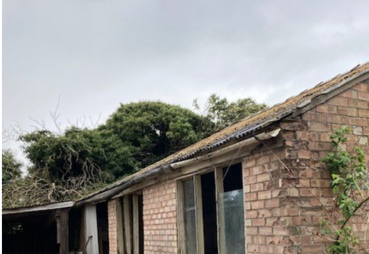
Dilapidated rainwater goods
