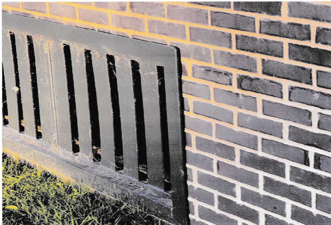
Photo of the grids approved by the EA to allow the flow of floodwater beneath the dwelling in the event that flooding should occur whilst preventing the access of detritus
