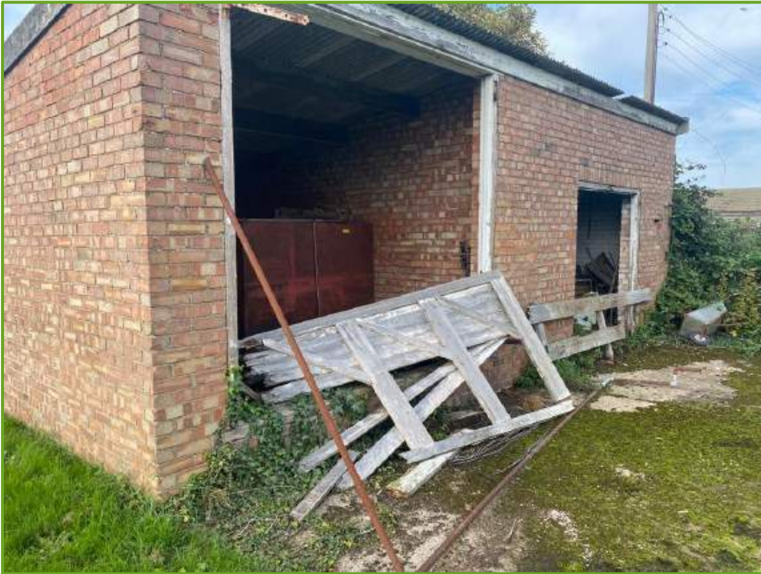
Photograph 5: Northern outbuilding - derelict.
