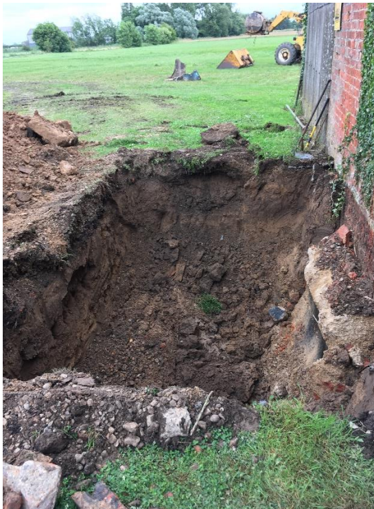
Remaining void following removal
