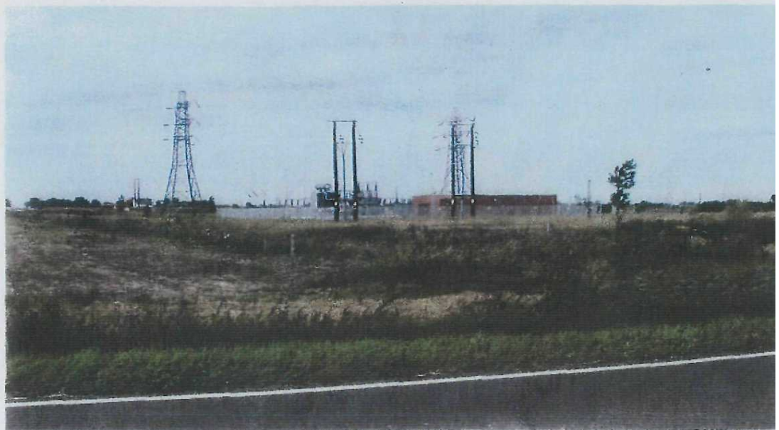
Power distribution infrastructure south of Holbeach
