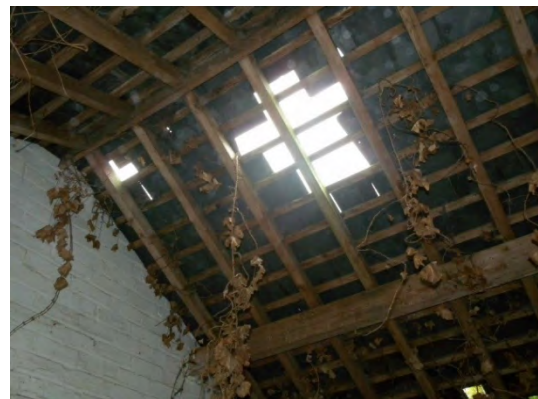
Photograph 9: Missing slates on northern small store
