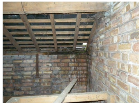
Photograph 5: Missing slate in south western corner of two-storey barn
