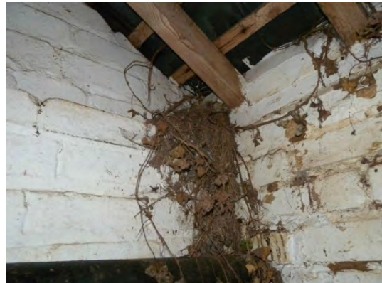
Photograph 28: Disused blackbird nest in northern small store
