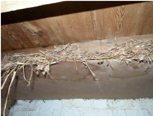
Photograph 25: Disused blackbird nests on ground floor of north-east two-storey barn
