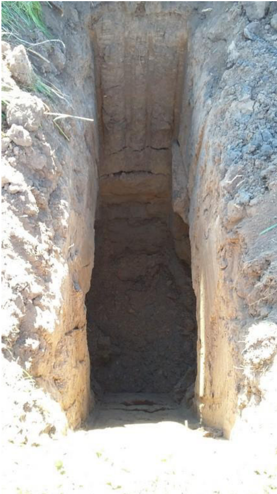
Photograph 7: Trial Pit TP4, showing the collapsing of trial pit sides due to saturated soil.
