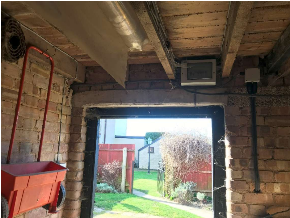
Photo 13. Store 2 lintel with minimal end bearing on RHS
