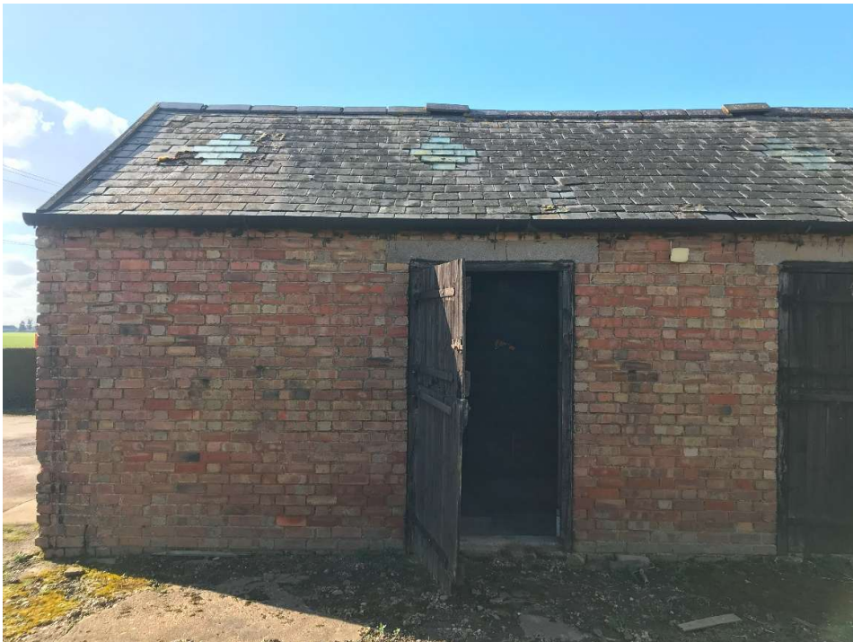
Photo 11. Store 1 cracked lintel from outside
