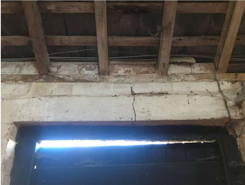
Photo 12. Store 1 cracked lintel from inside
