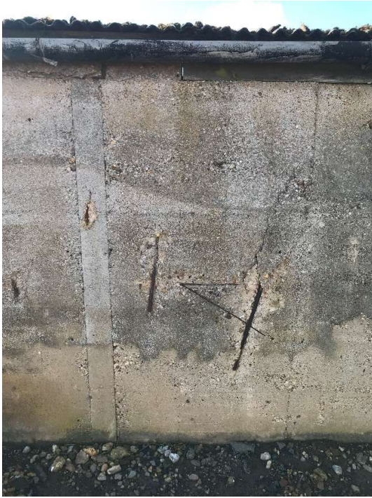
Photo 24. Store 5 load bearing RC wall with exposed reinforcement
