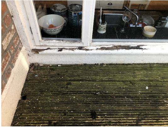
Extent of damage to kitchen window (W1)
