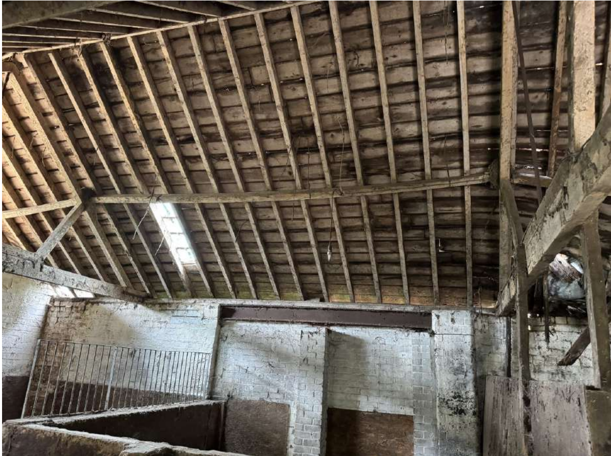
Image 8.0: Interior of long span bay showing steel beam to rear elevation and internal stable partitions. Purlin to mid-span of rafters is overstressed and has sagged excessively.
