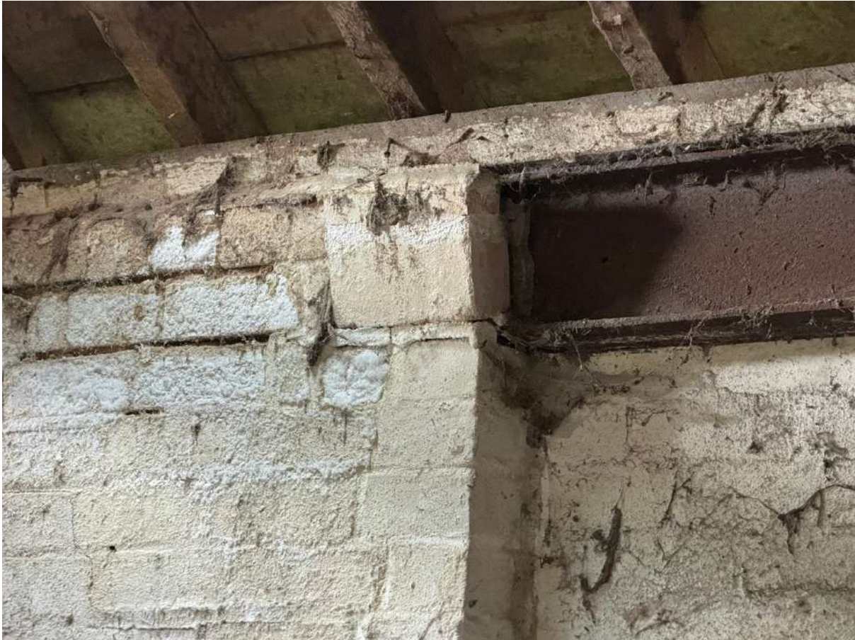
Image 9.0: Masonry and beam rotating outward due to thrust imparted to head of wall panel by rafters.
