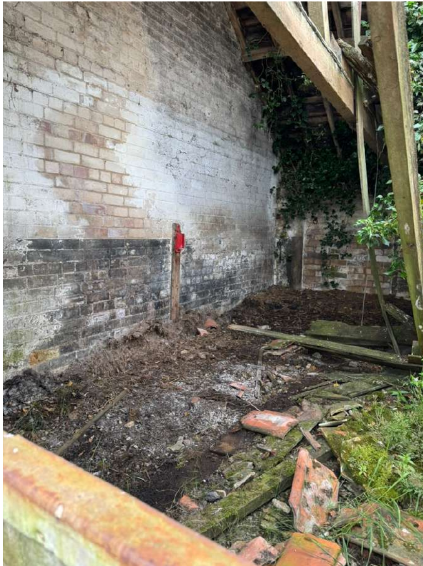
Image 4.0: Horse muck, rising to approximately 1 meter above finished floor level. Collapsed roof with remaining truss
