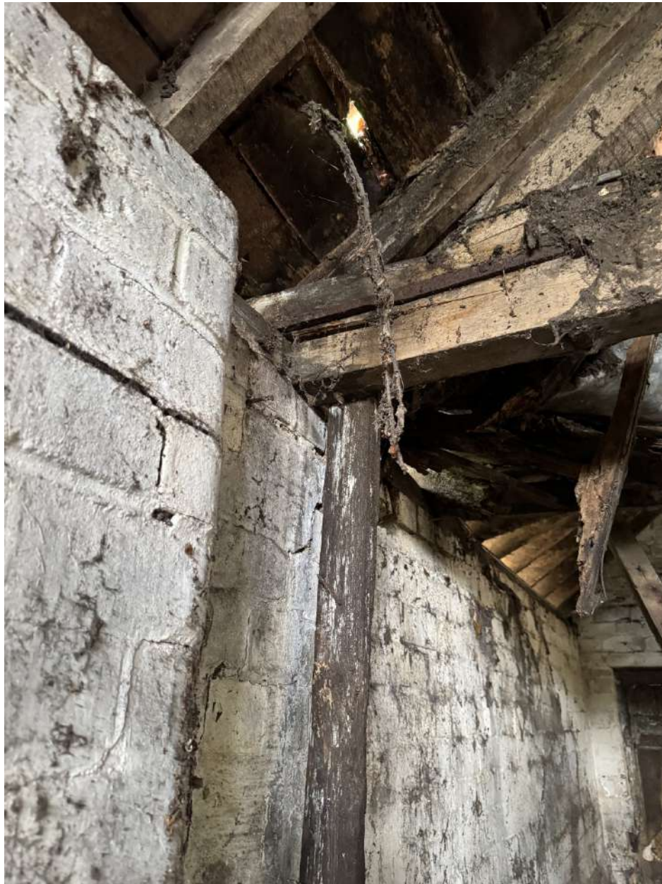
Image 10.0: Collapsed valley junction and split truss, now supported on timber post
