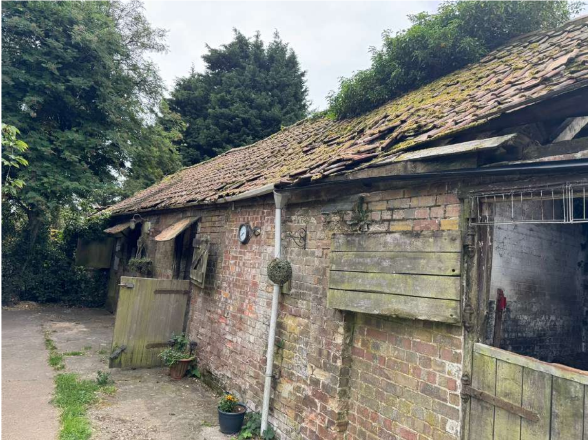
Image 12.0: Deteriorating roof structure, with tiles lost or dislodged, roofline wandering at ridge due to spread at eaves.
