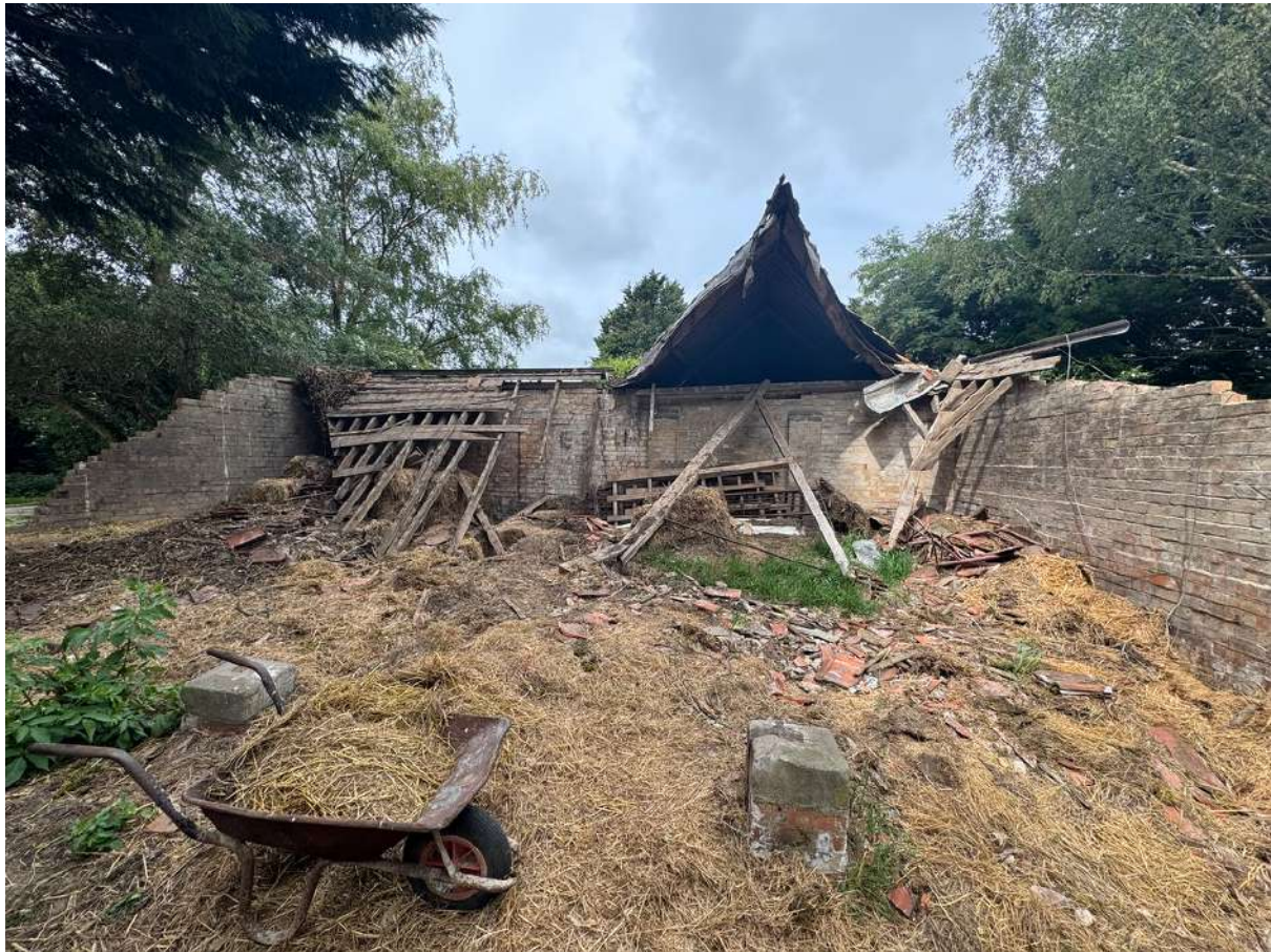
Image 11.0: Collapsed end of barn structure
