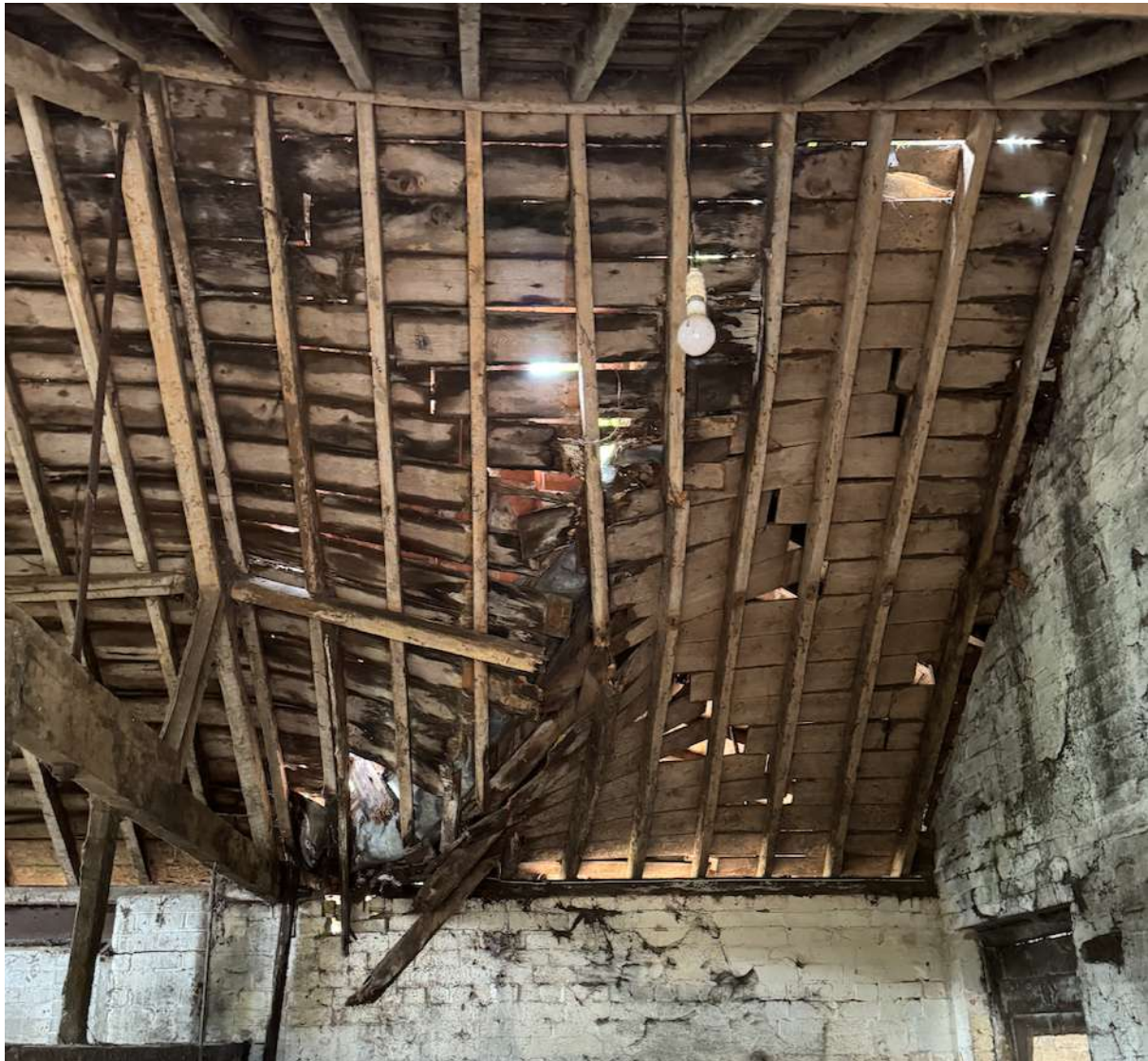
Image 7.0: Failed purlin, rafters, valley to adjacent roof, failed sarking boards and deflecting ridge board.
