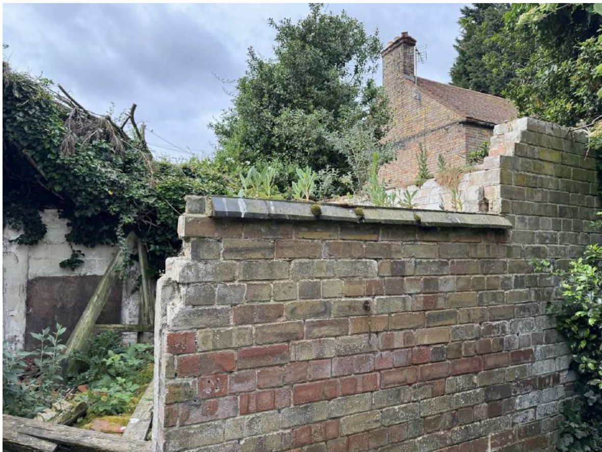
Image 3.0: Collapsed section adjacent to main residential property, gable and side walls standing
