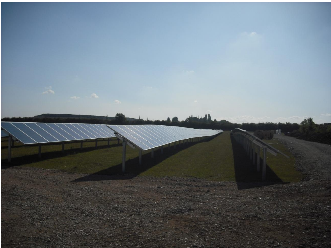
Similar but larger PV array
