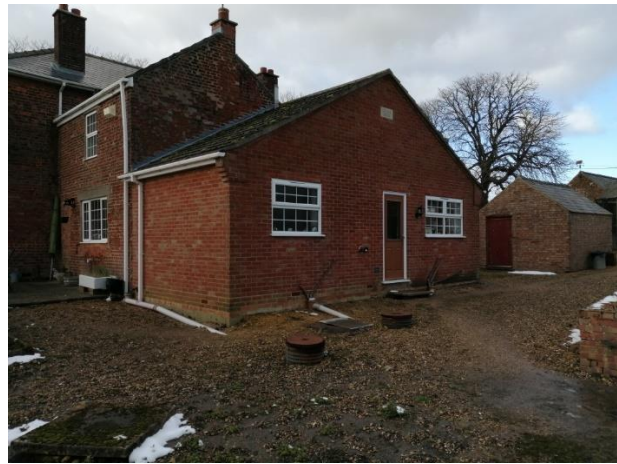
Existing rear elevation showing extension and poor brickwork to upper storey
