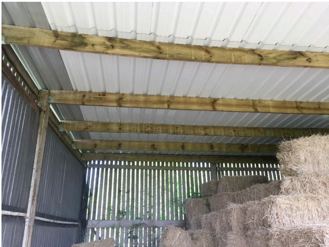
Image 10.0: Excess deflection to rafters over rear Section of structure.
