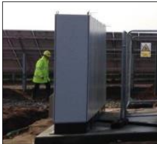
EXAMPLE: MARSHALLING CABINET / COMBINER BOX ON SITE
