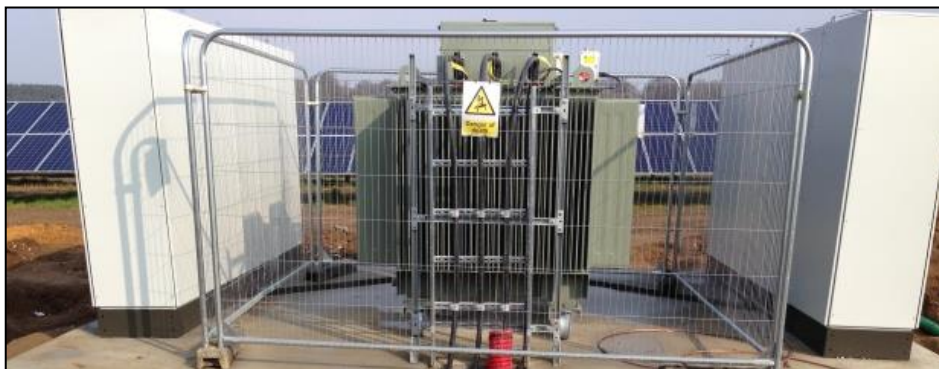
EXAMPLE: TRANSFORMER ON SITE
